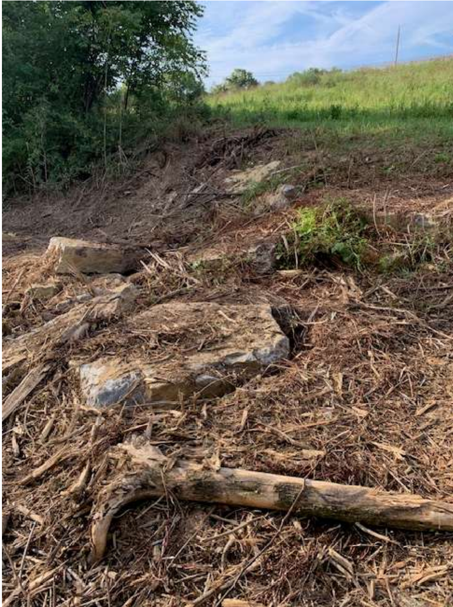
Displaced rock armor and, upper left, at a gouged-out stream bank
