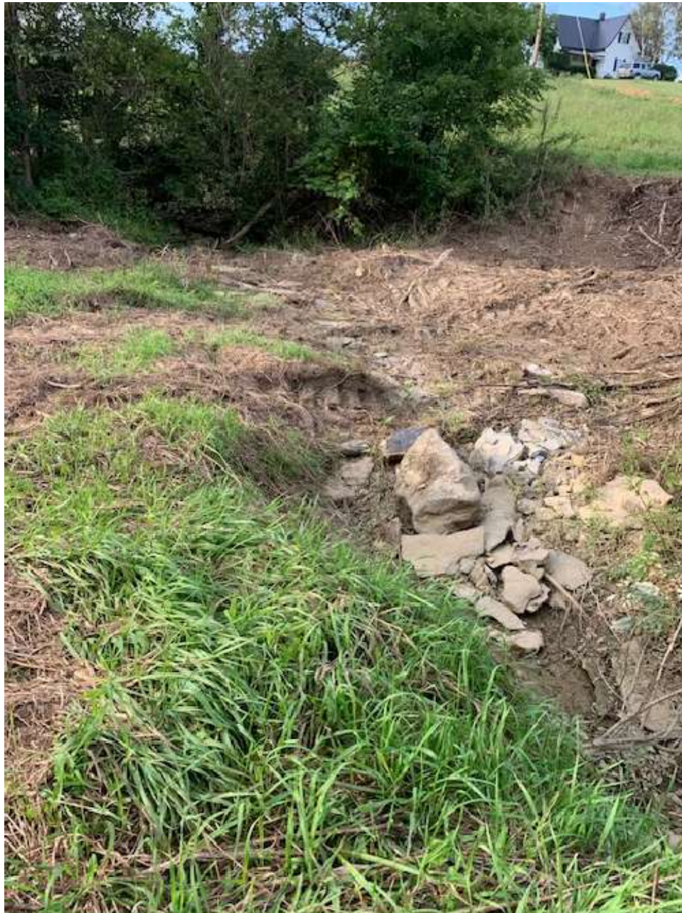
Unauthorized stream modification contributing to storm water backup and flooding of neighbor's yard threatening or flooding his water meter
