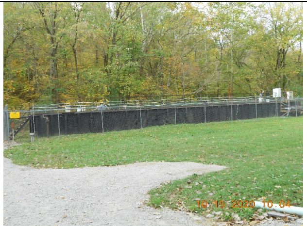
Same chemicals and more improperly stored
