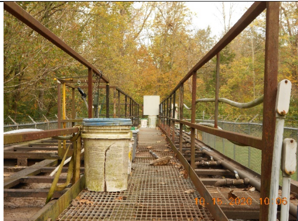
See no repairs to walkway
