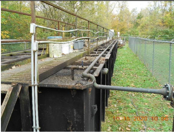
No air jet valves in full open position.
