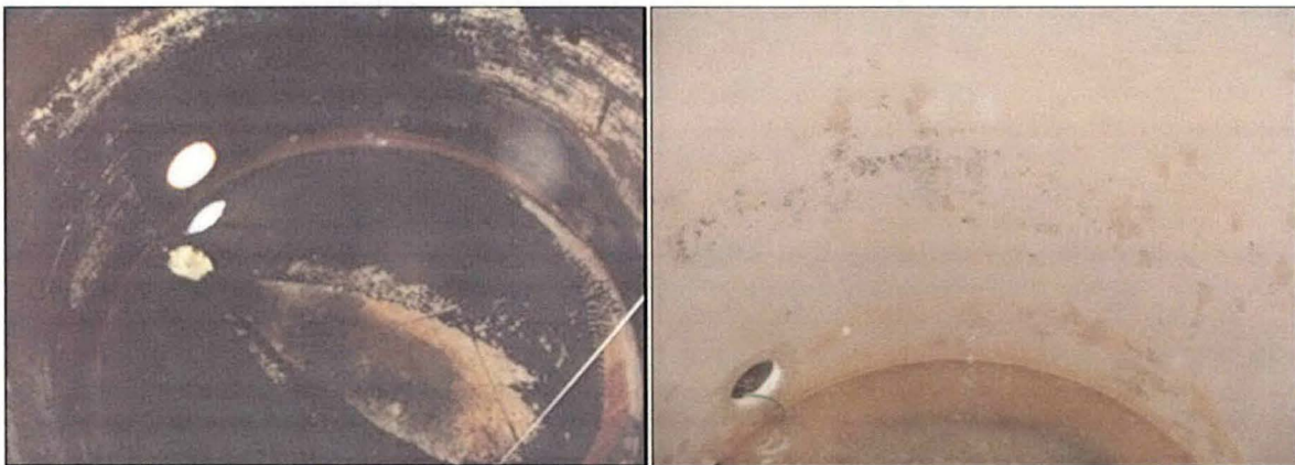
Figure 2: The Oklahoma clearwell prior to chemical cleaning (left) and after cleaning (right). Biofilm and accumulated deposits were removed exposing areas of corrosion.
