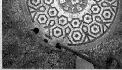
Open Pick Hole in Casting
