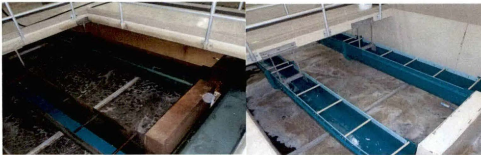
Figure 3: The spray-on/rinse-off chemical cleaning solution makes it easy to remove unsightly surface stains from filter basins.
