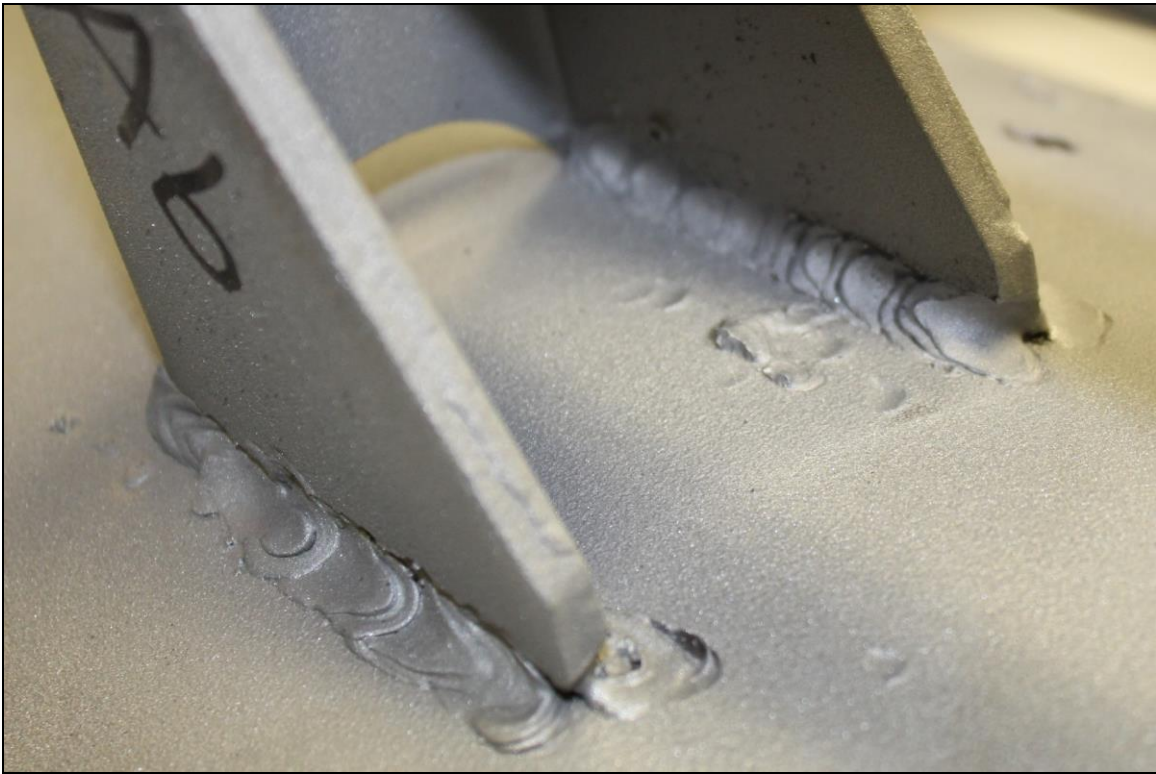
Figure 9. Image of the Lug A6 exterior top and interior bottom welds which exhibited substantial fusion except for some undercut, arc strikes, and porosity.
