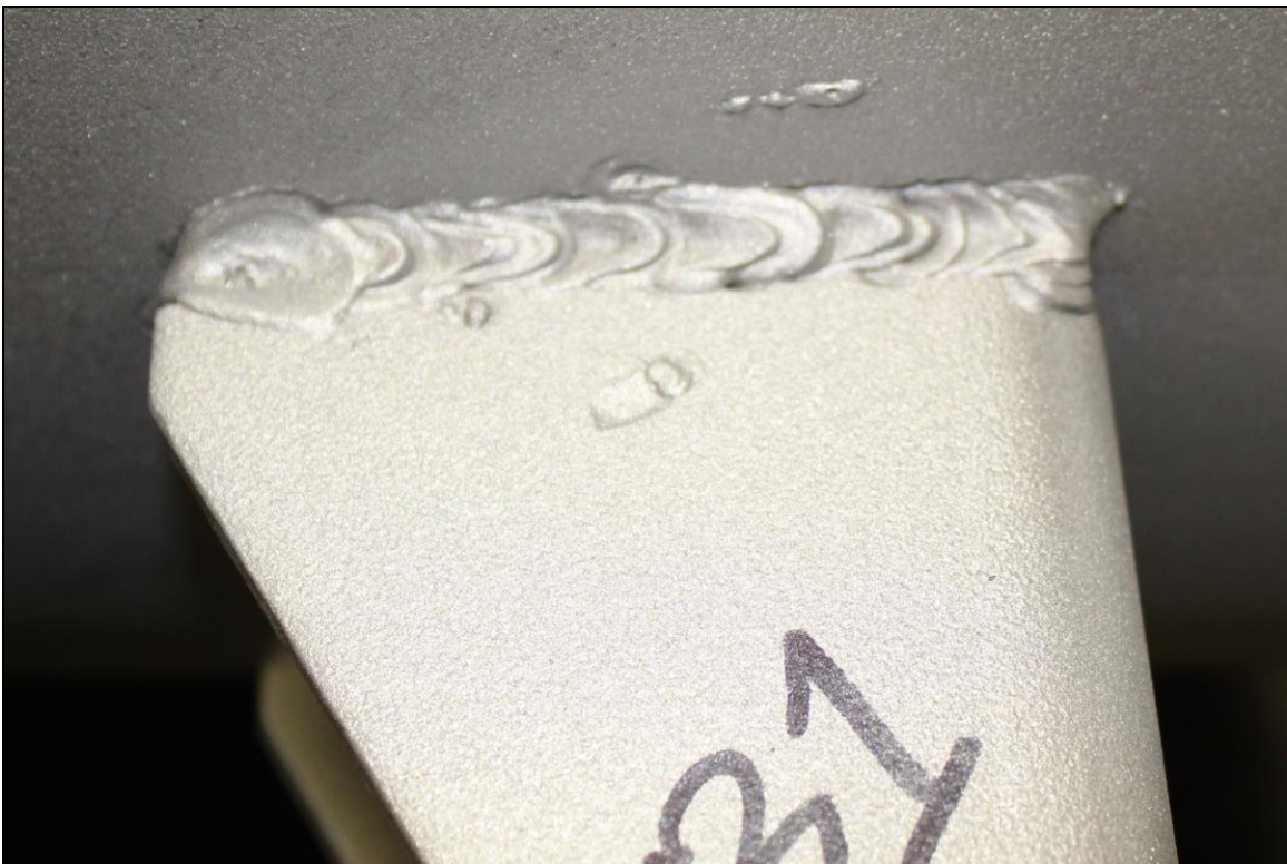
Figure 10. Image of the Lug B1 exterior top weld which exhibited substantial fusion except for arc strikes, undercut, and spatter.
