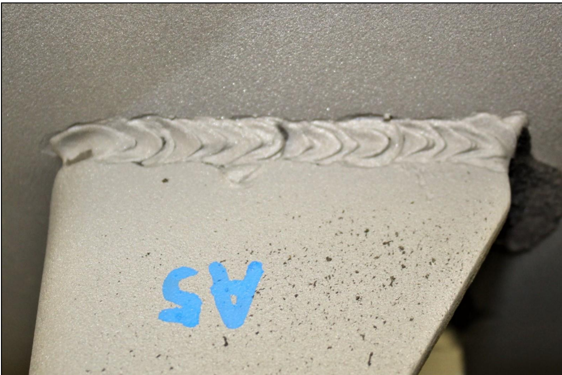
Figure 8. Image of the Lug A5 exterior bottom weld which exhibited substantial fusion except for some undercut and porosity.
