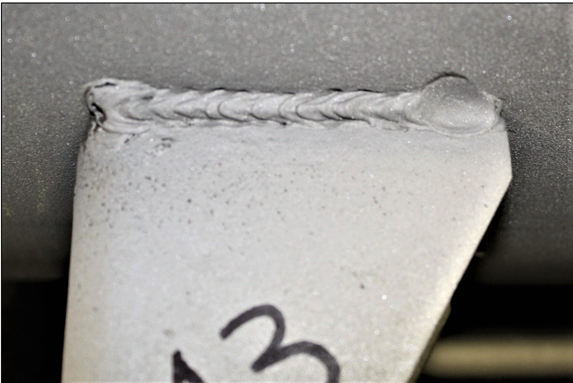
Figure 6. Image of the Lug A3 exterior top weld which exhibited substantial fusion except for some undercut and porosity.
