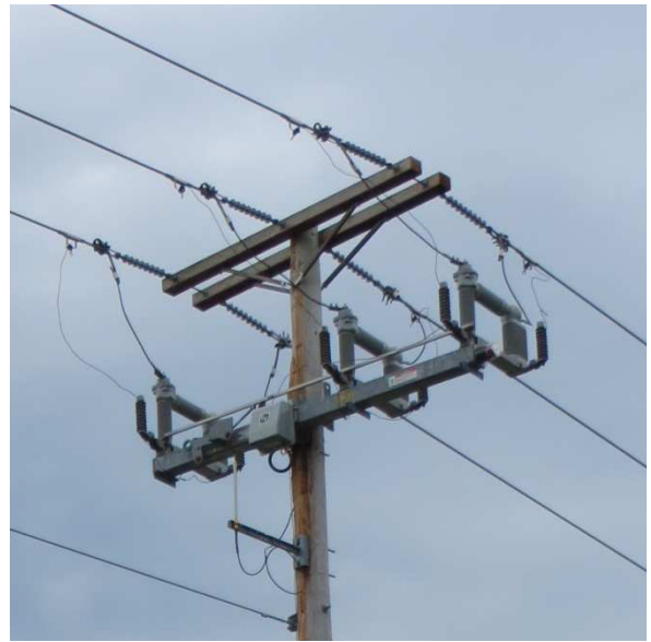
Automated switches mounted to utility poles can be used to create self-healing grids that improve reliability by isolating faulted sections of the distribution system.
