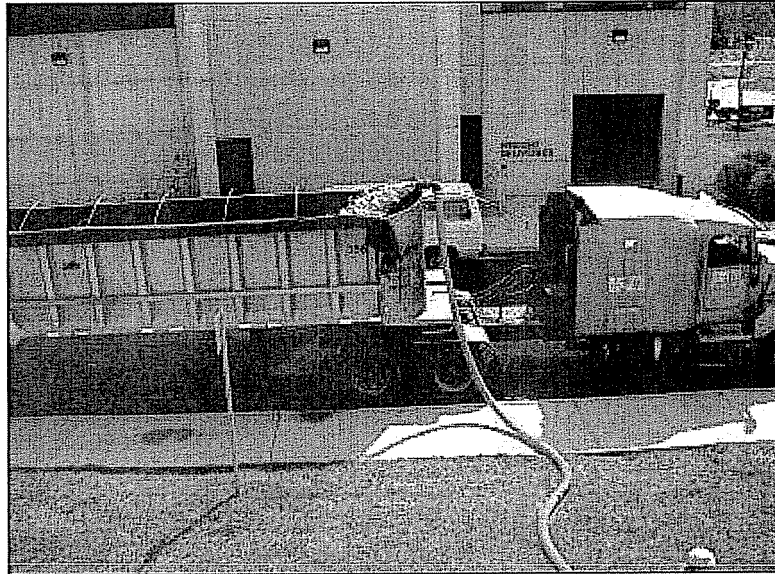
EXHIBIT 5-29 Media Removal by Eduction to Open-Bed Truck (Provided by Calgon Carbon Corporation)
