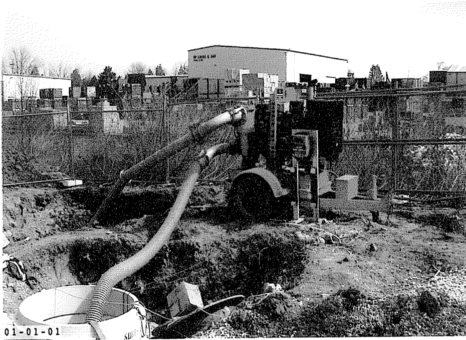
Bypass pump and bypass valve
