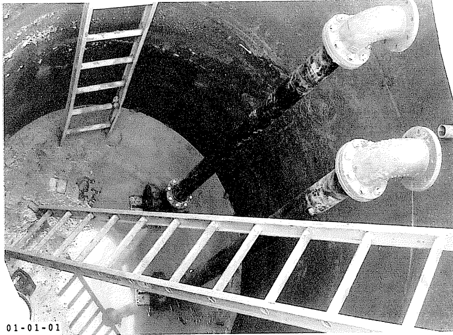
New discharge lines and valves
