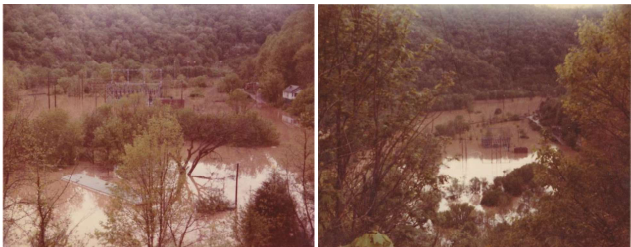
Photos 1 and 2. Flooding of Allen Substation (1984)
