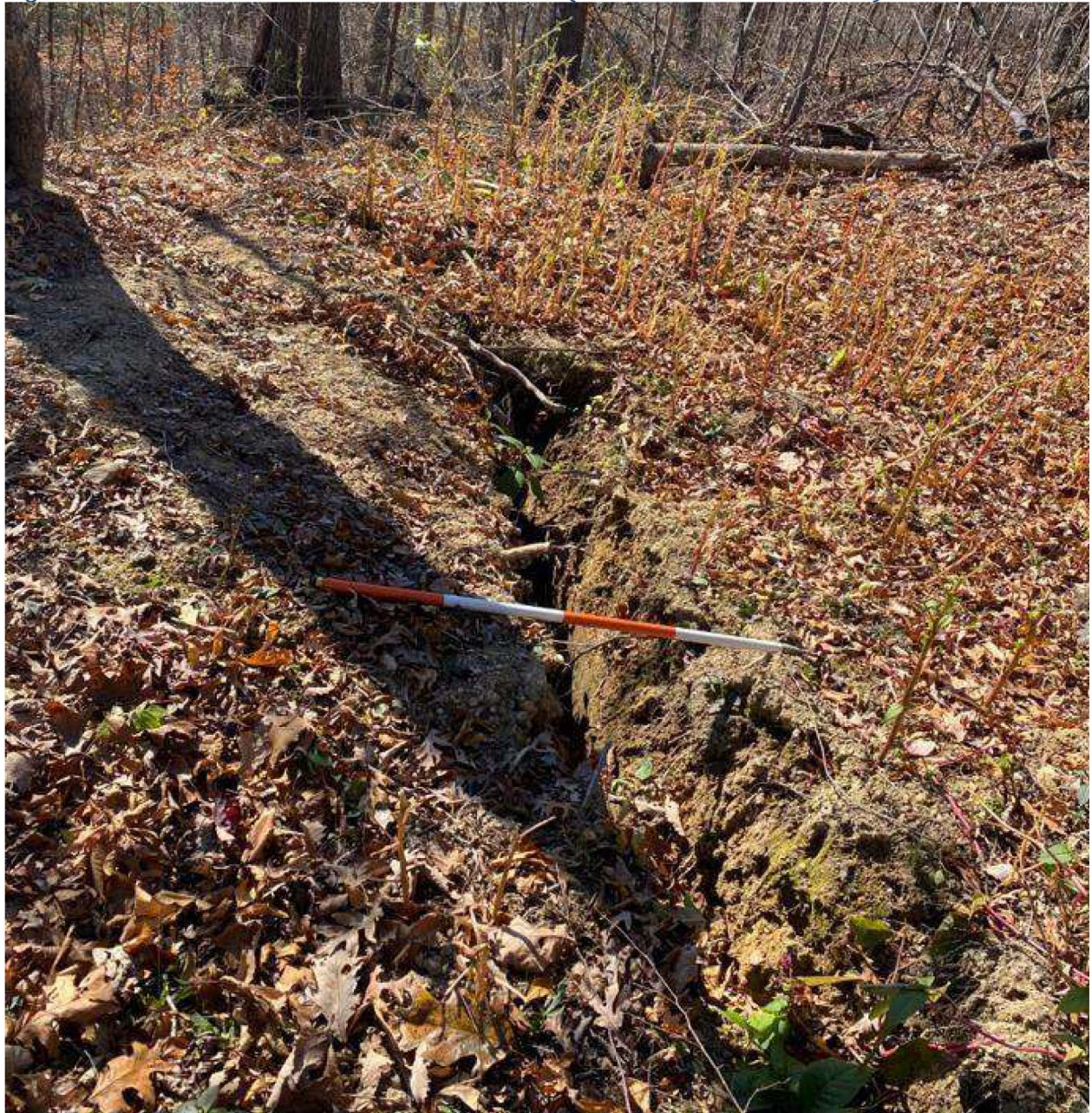
Figure 1 Mine Crack Across Access to Str 5 and 6 (dated November 17, 2021)
