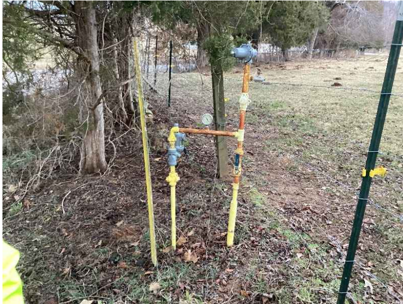
PHOTO 7: REGULATOR STATION ALONG IRVINGTON BEWELYVILLE ROAD
