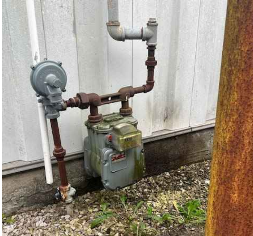
PHOTO 9: TYPICAL CUSTOMER METER.
