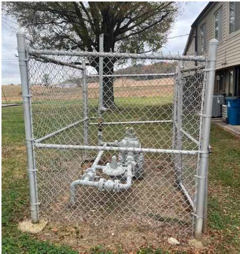
PHOTO 8: METER LOCATED AT HOUSING DEVELOPMENT.
