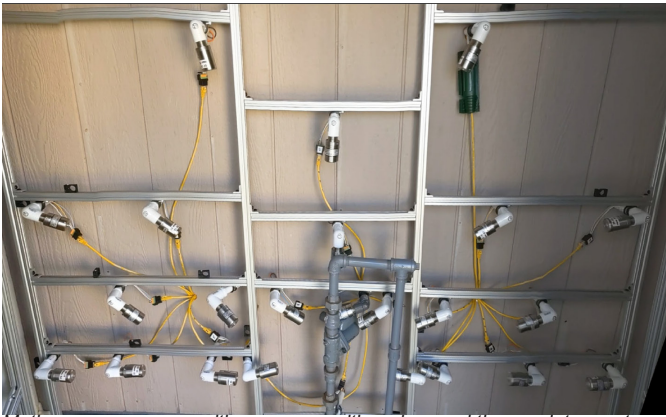
Methane sensor array with sensors positioned around the regulator vent.
