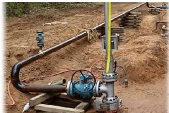
A below-ground pipeline section that has been isolated using stopples and an above-ground bypass line to avoid service interruption to customers
