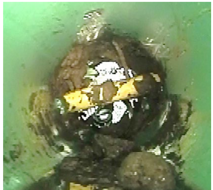
Blockage caused by Cross-Bore in Sewer Line
