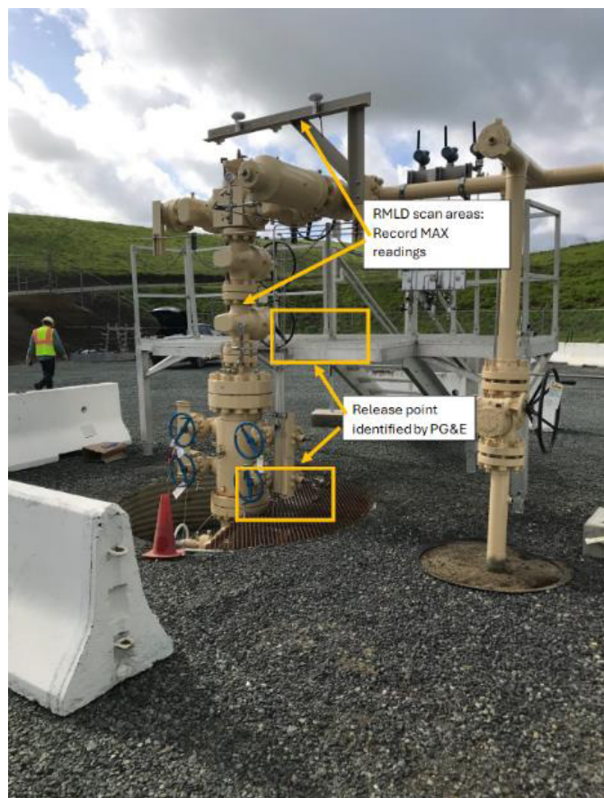
TEST SET-UP IN THE UNDERGROUND STORAGE FACILITY
