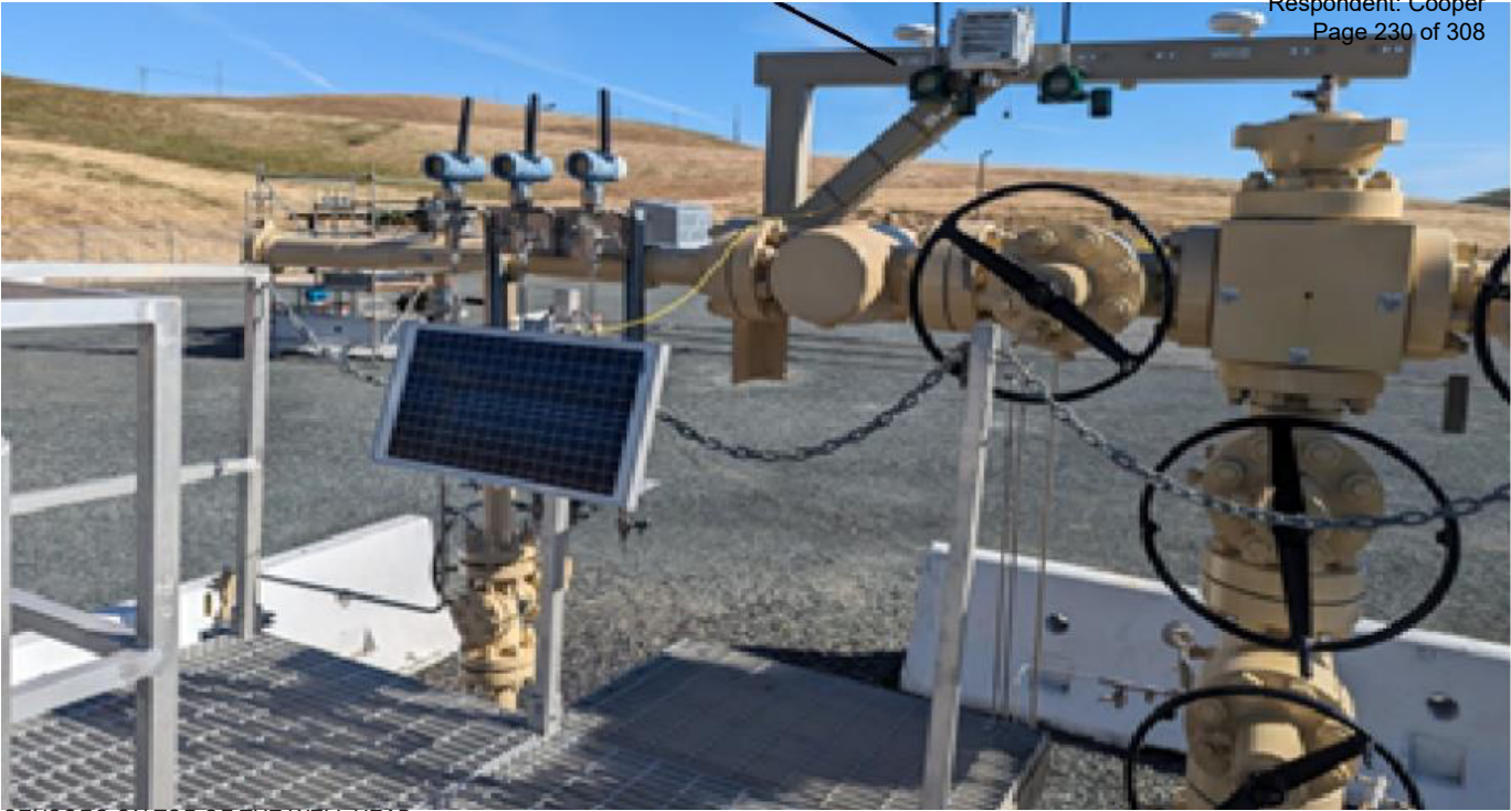
SENSORS ON TOP OF THE WELL HEAD
