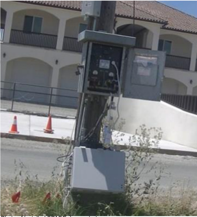
Photo of installed SPADE demonstrator
