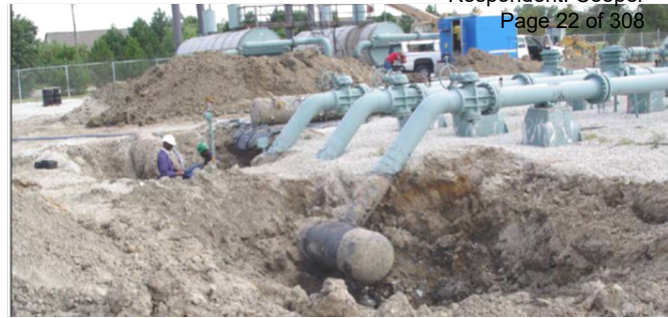
Congested meter-regulator station DA site with tees, stubs, and tap lines.
