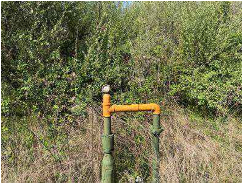
View of a gas well on the western portion of the Subject Property (Lexington Coal parcel 030-00-00-047.00).
