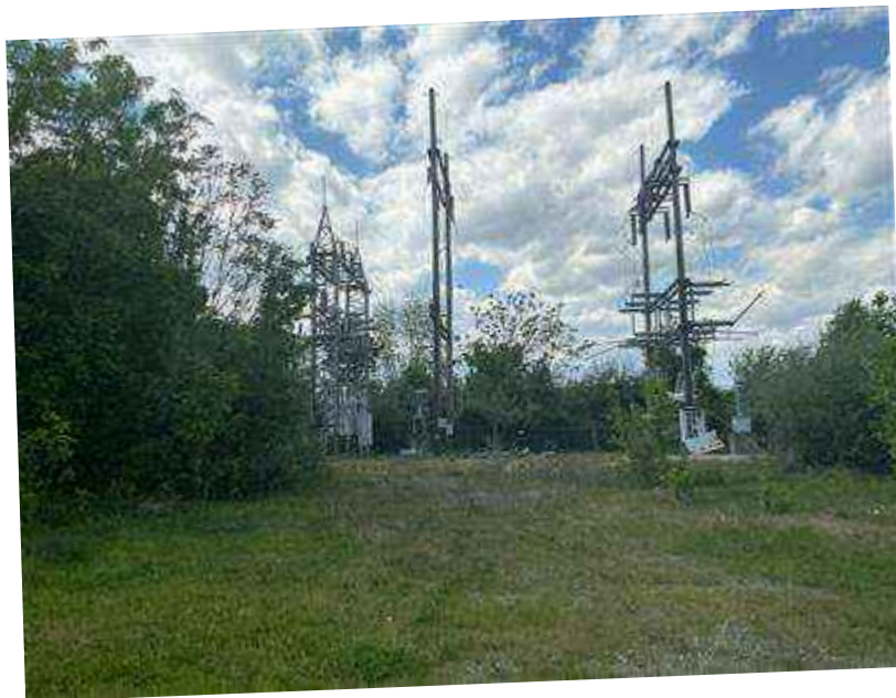
View of a substation and tote to the south of Pocahontas parcel 040-00-00-020.00.
