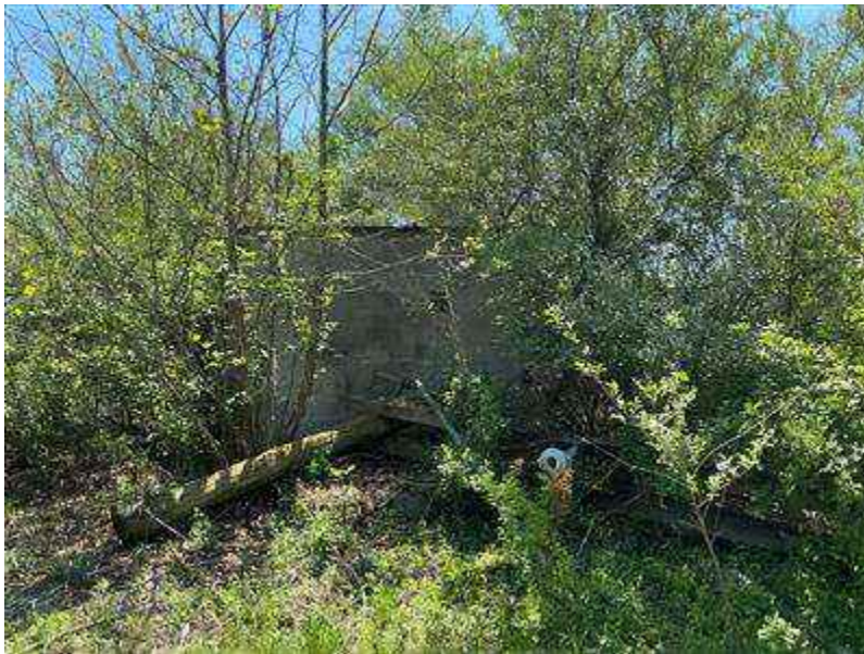
View of a dilapidated structure on the eastern portion of the Subject Property (Pocahontas parcel 040-00-00-020.00).
