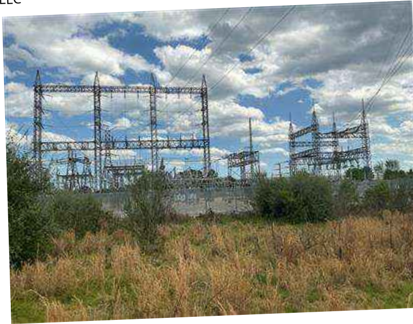
View of a Substation to the south of Pocahontas parcel 040-00-00-020.00.
