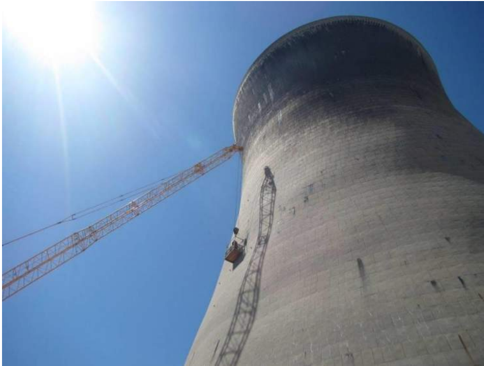
Photo 3. Visible distorted shape of the concrete shape
