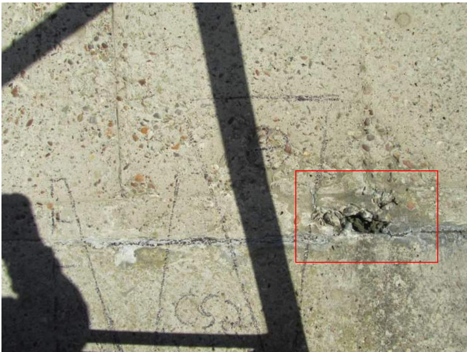
Photo 7. Unconsolidated concrete at a construction joint
