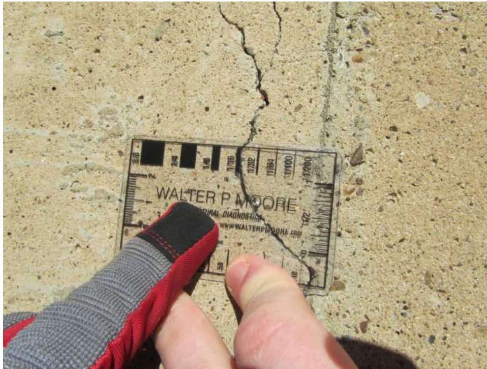
Photo 5. Close-up view of a crack in concrete veil
