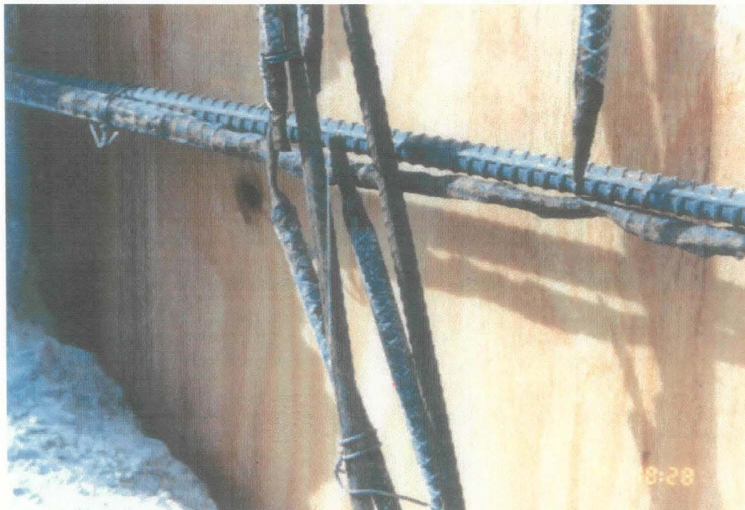
Reinforcement with corrosion - induced section losses
