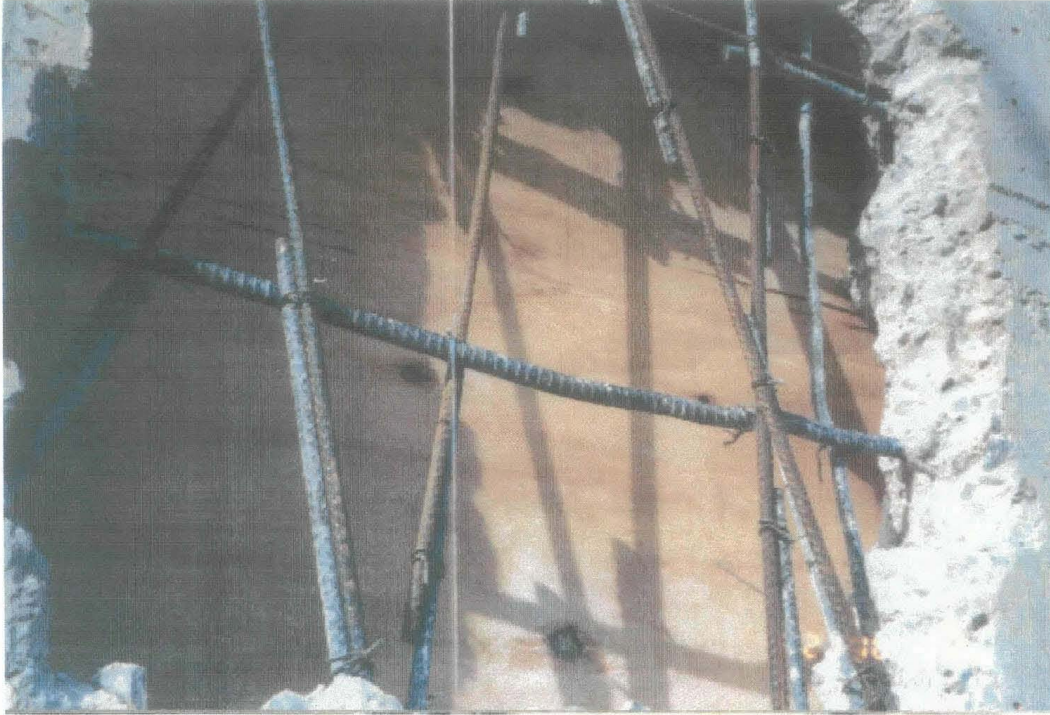
Exposed reinforcement from concrete removal
