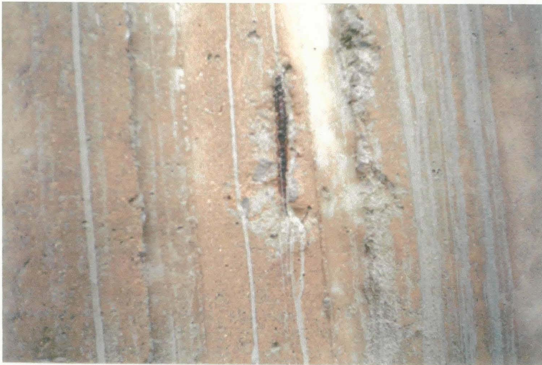
Specimen Photograph No. 12 Corroded rebar
