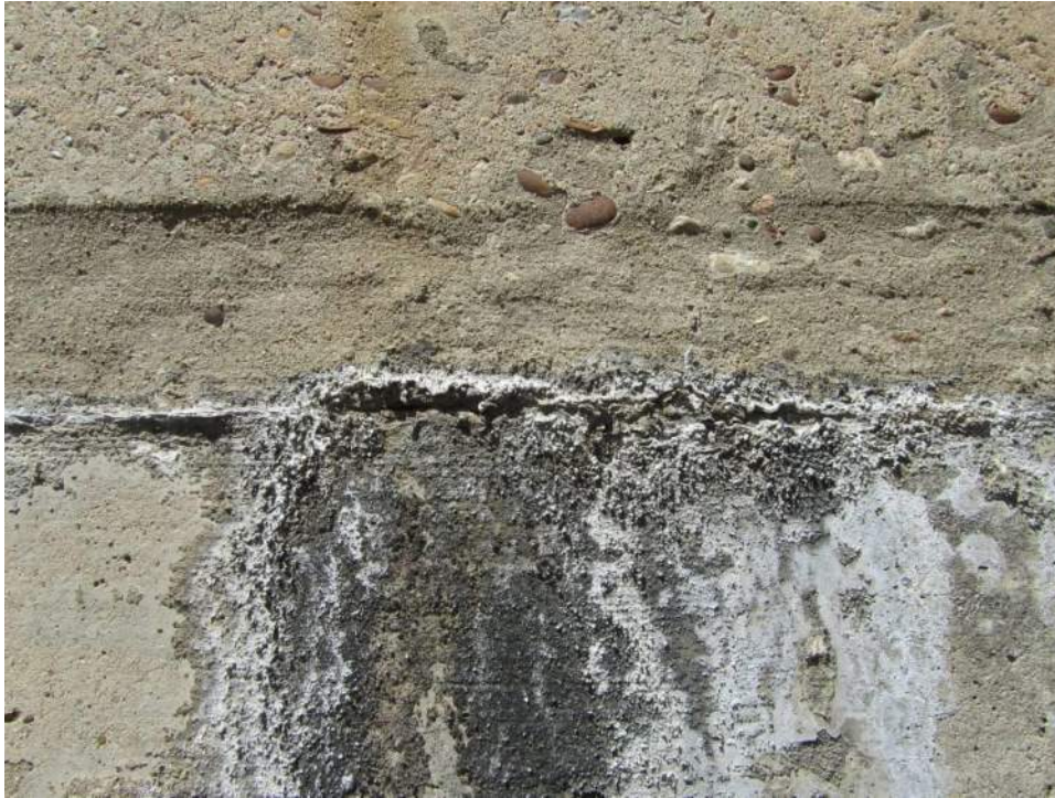
Photo 9. Efflorescence at a construction joint
