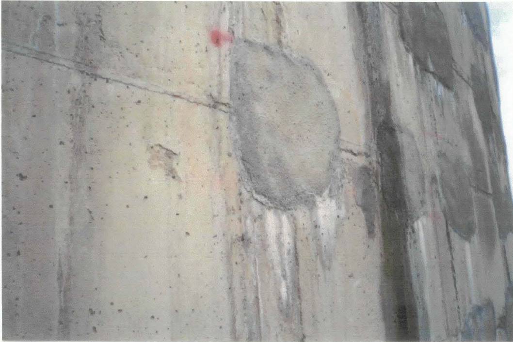
Specimen Photograph No. 9 Patch repairs on exterior face of Cooling Tower Shell. Note efflorescence and water leakage conditions along patch perimeter
