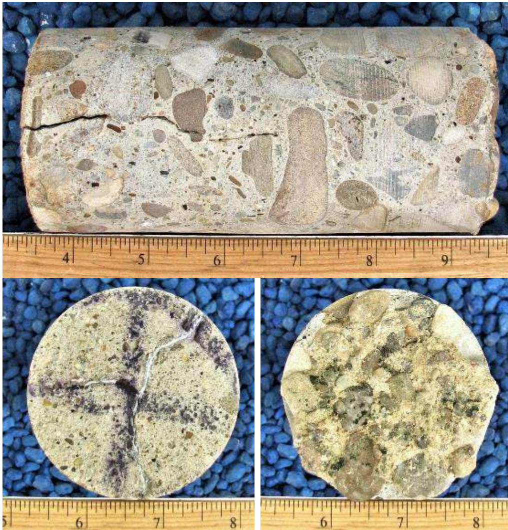
Figure 1 – Core CP1 as received for examination (exterior surface oriented to the left).
