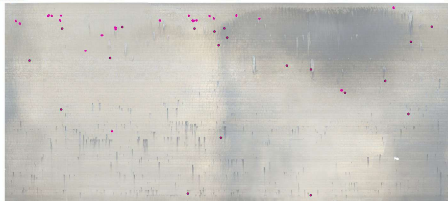
Defects with falling risk N - W - S - E - N
