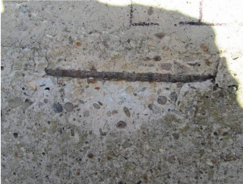
Photo 7. Concrete spall and exposed reinforcement
