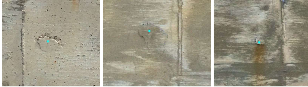
Defects with falling risk
