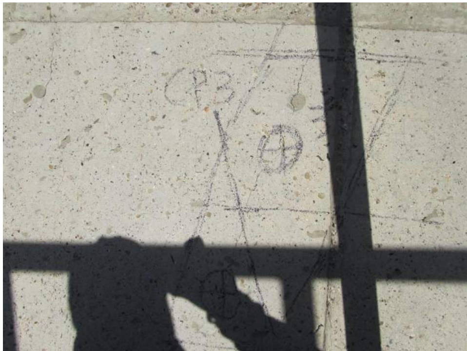
Photo 6. Location marked for a petrography core crossed by a crack
