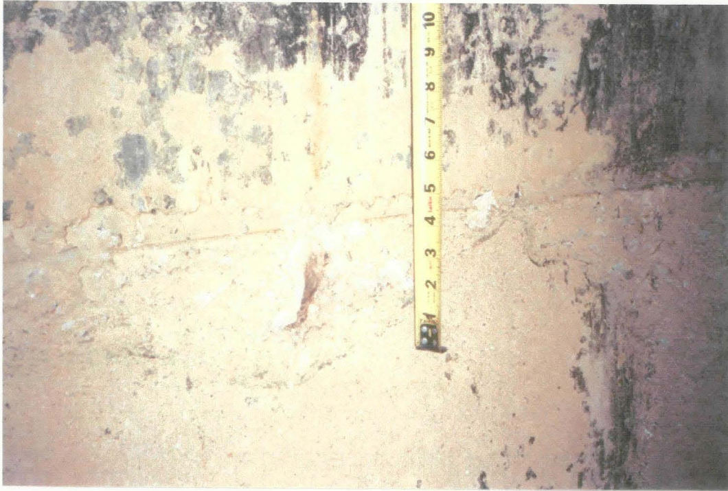
Specimen Photograph No. 11 Typical honeycomb at panel joint locations
