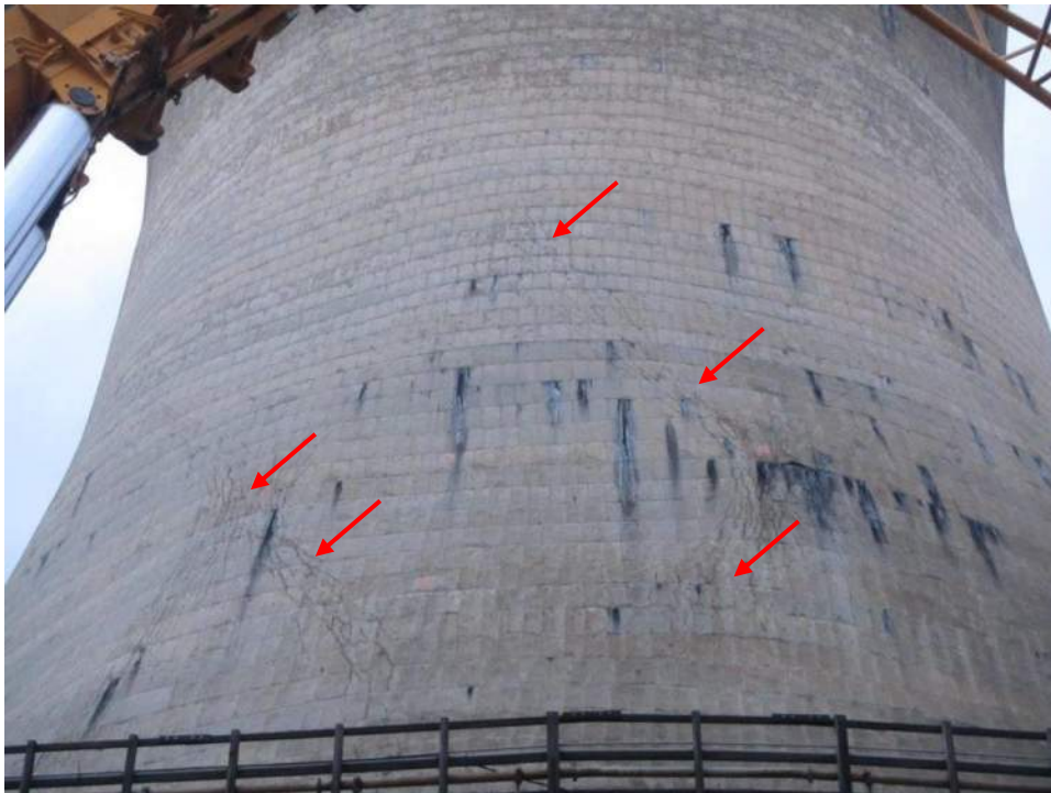
Photo 4. Visible cracking in the concrete veil
