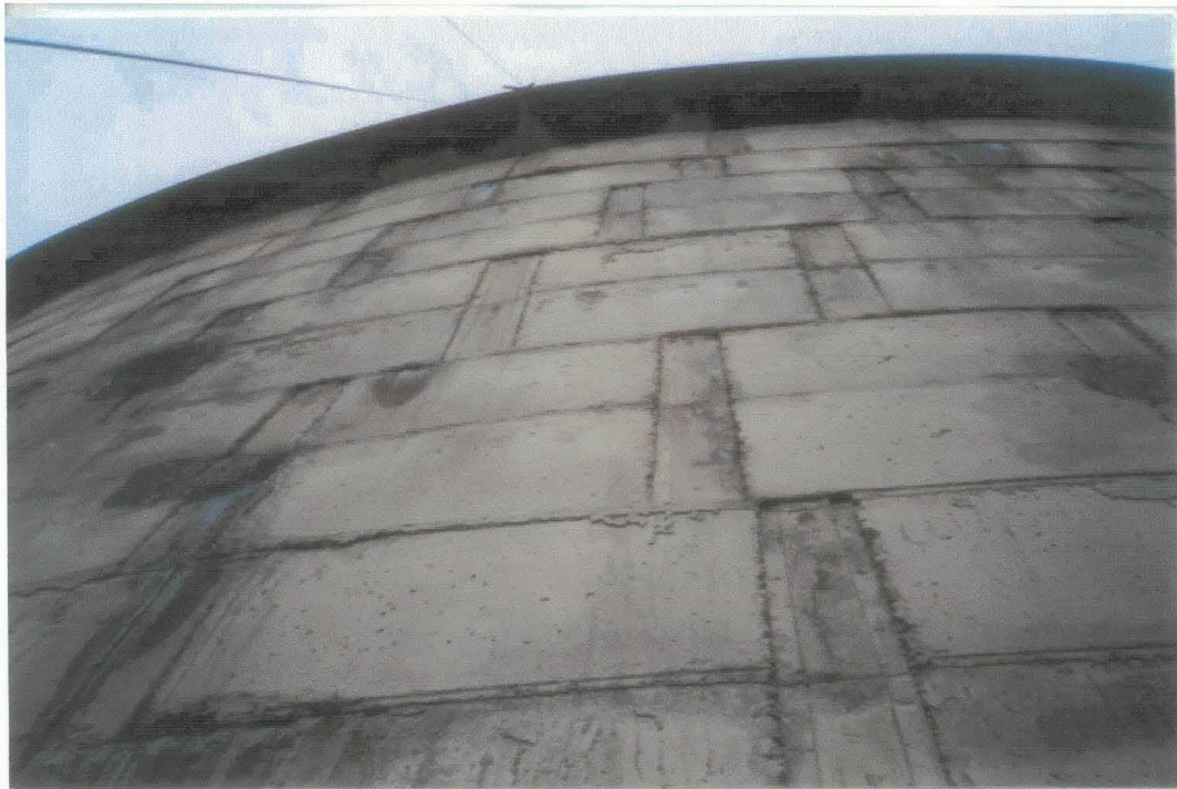
Site Photograph No. 8 Patch repairs and close-up of jump panel formwork impressions on exterior face on Cooling Tower Shell
