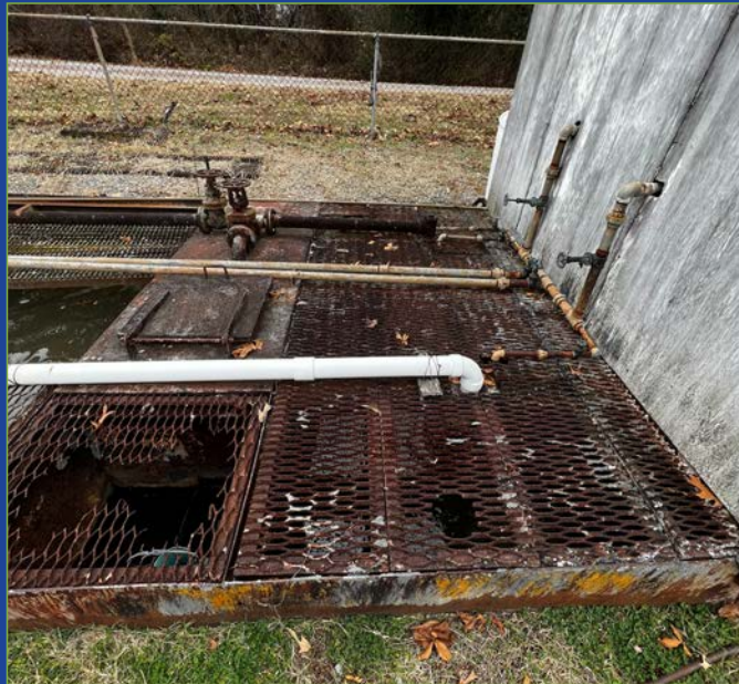
Rust at the Clarifier
