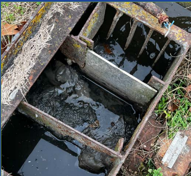
Ineffective spacing between bars on screen
