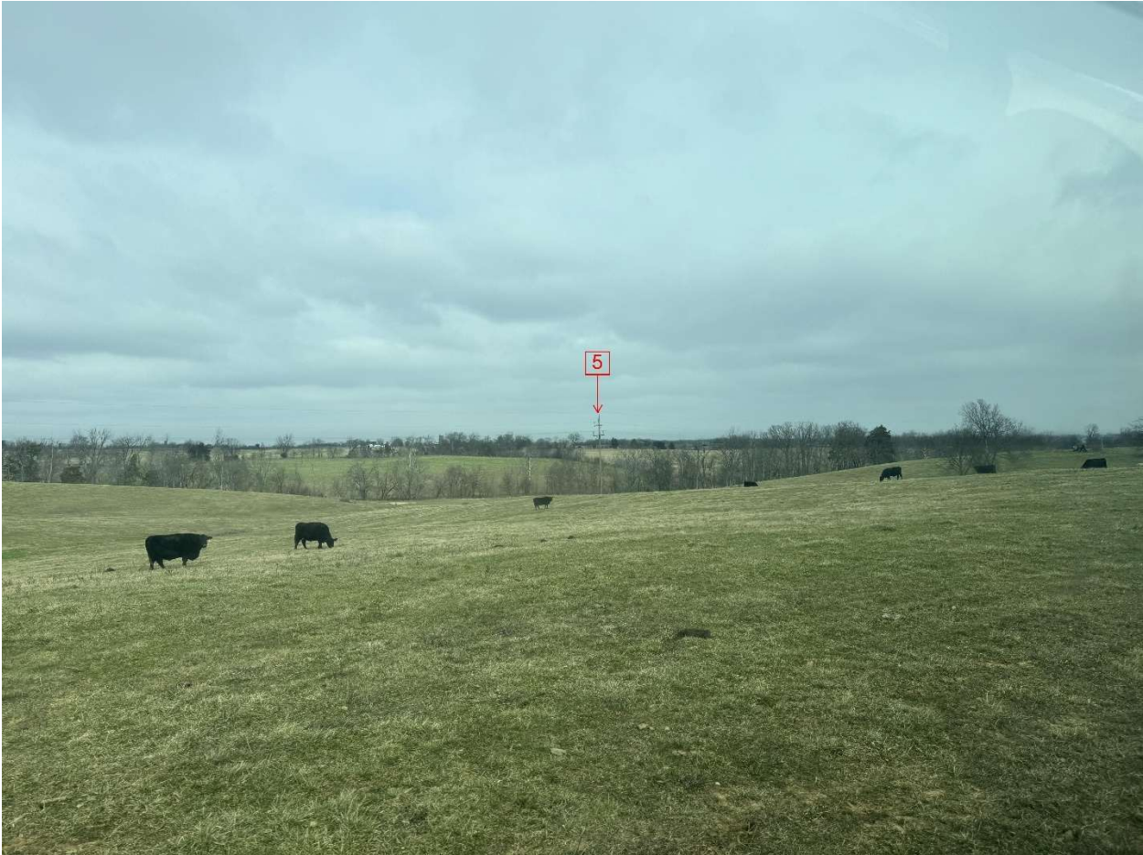
Figure 39 - Stop 4 – View 1, Sulphur Creek to Loretto 69kV EKP pole 5
