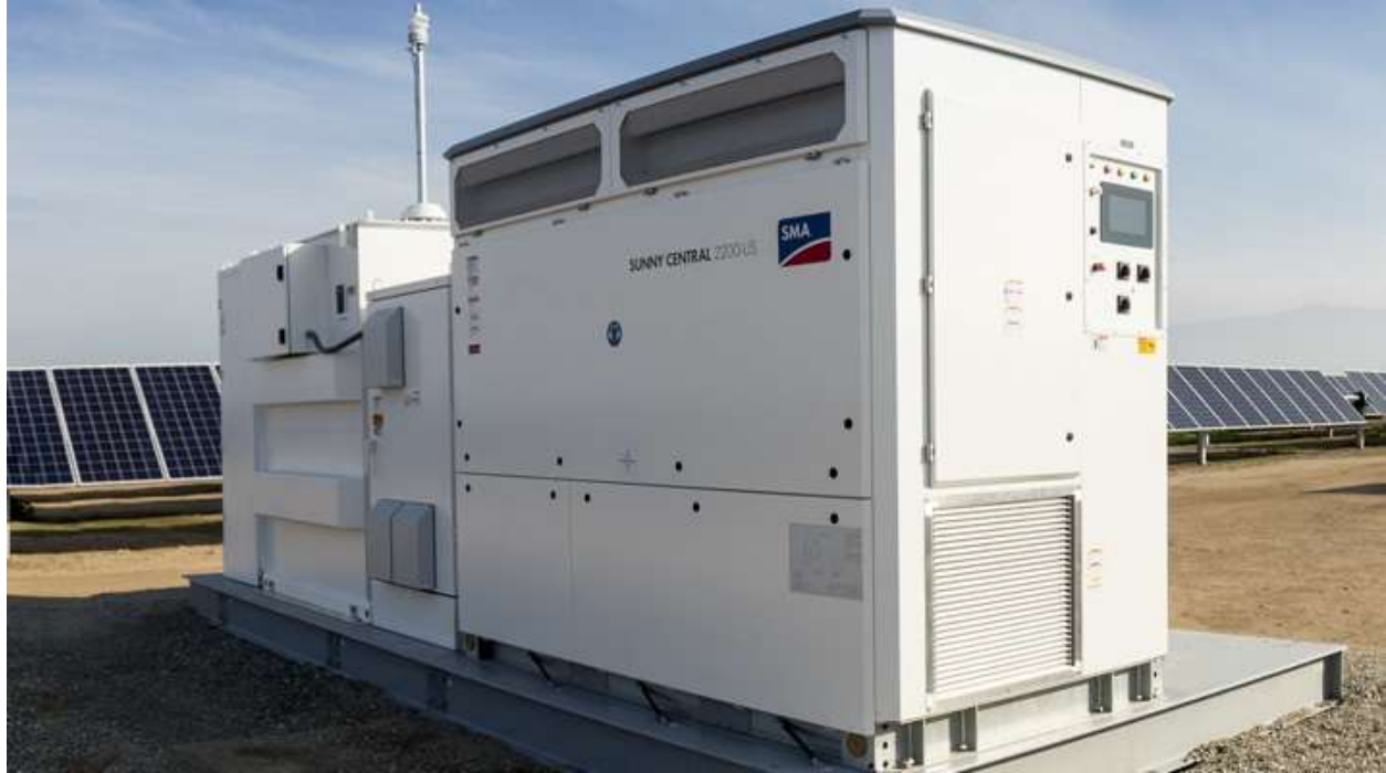
Picture (4) Industrial Solar Inverter 4
