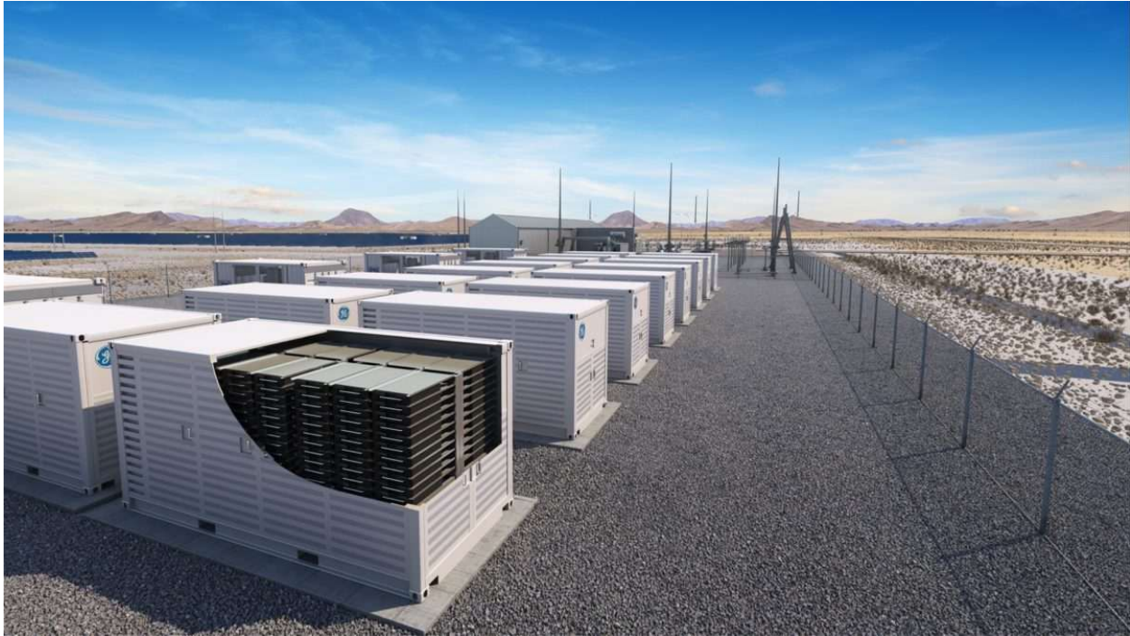
Picture (5) GE Industrial Battery 5
