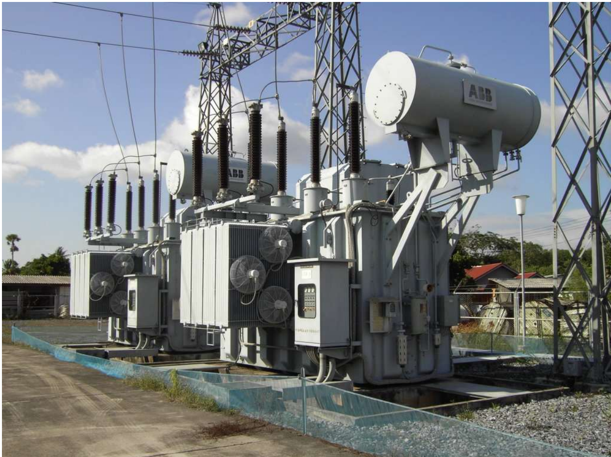
Picture (6) Substation Transformer 6
