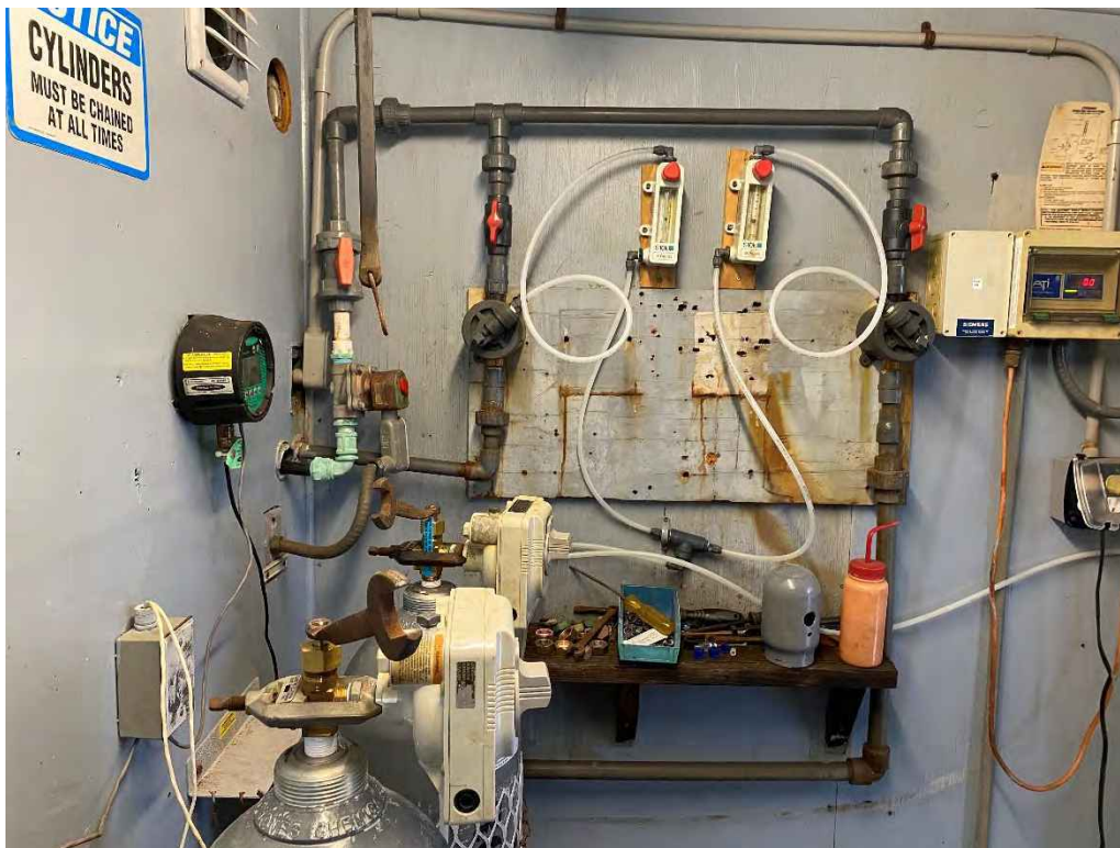
Chlorination Feed System
