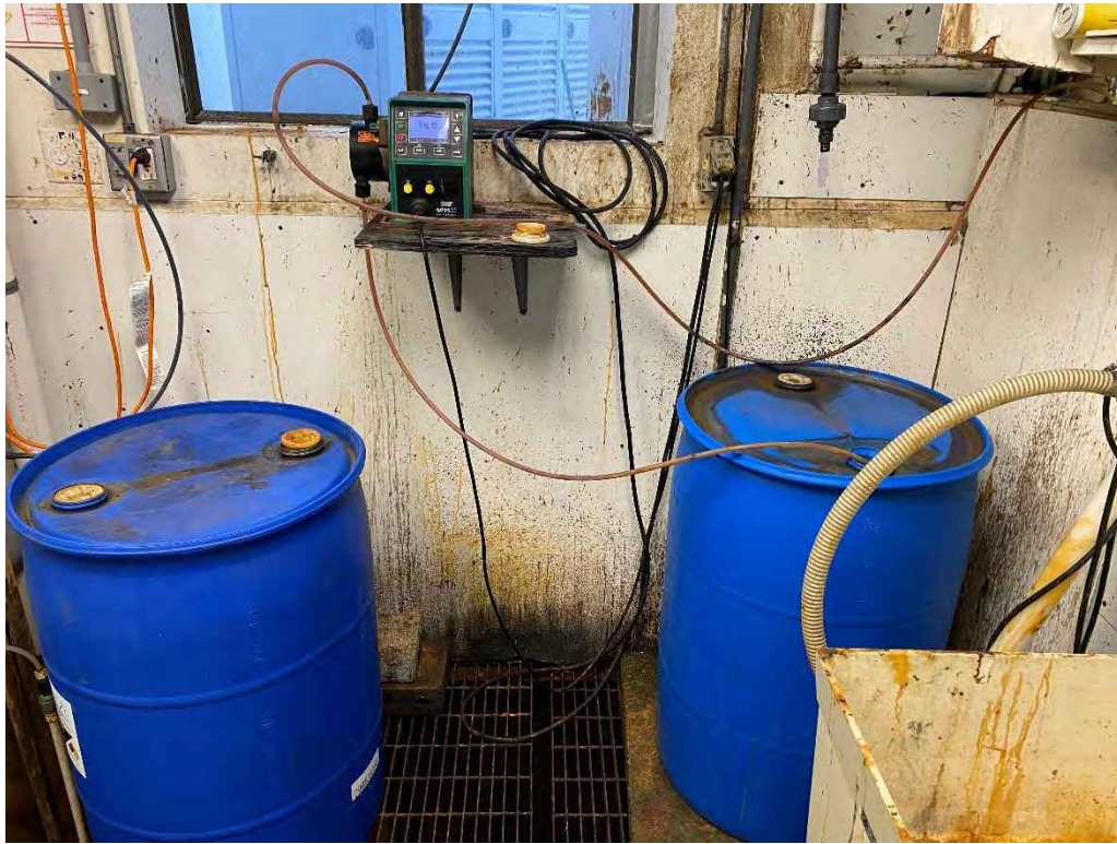
Chemical Feed System
