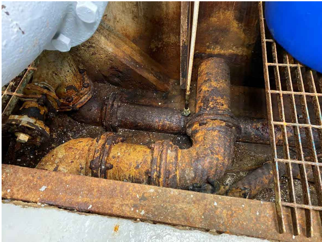
Raw Water Piping and Valves w/Chemical Feed Connection
