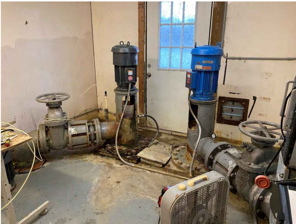
Vertical Turbine Raw Water Pumps
