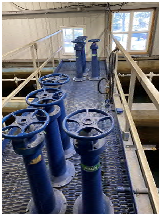
Filter Valve Operators
