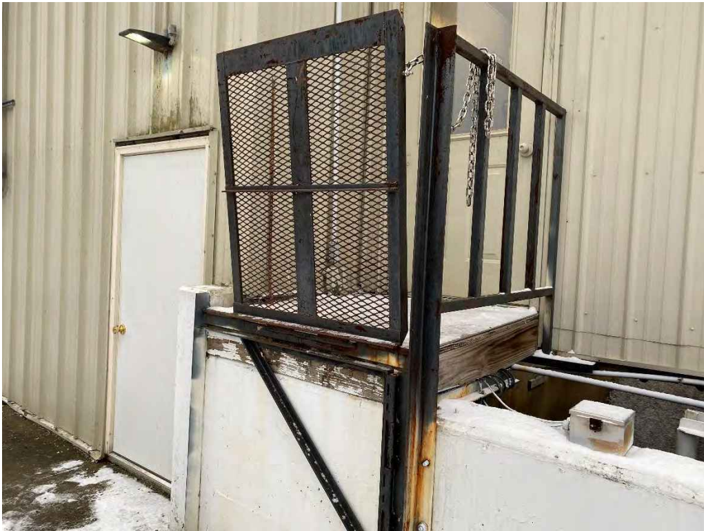
Chlorine Cylinder Lift and Access to Bldg.
