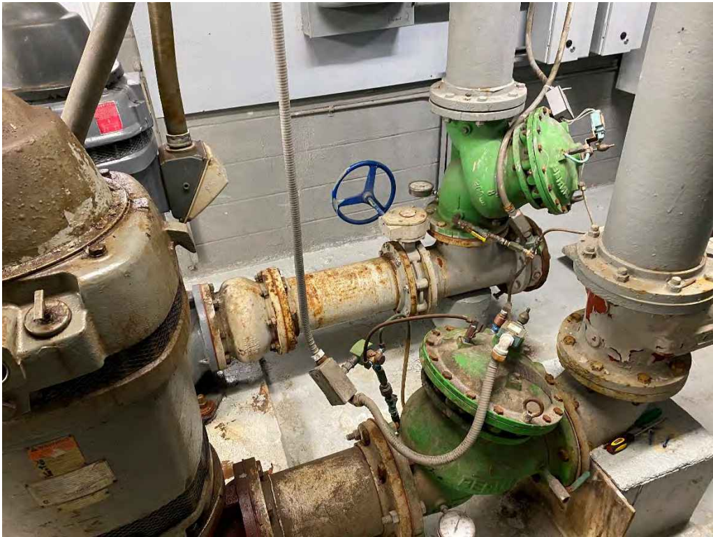
High Service Pumps and Valves
