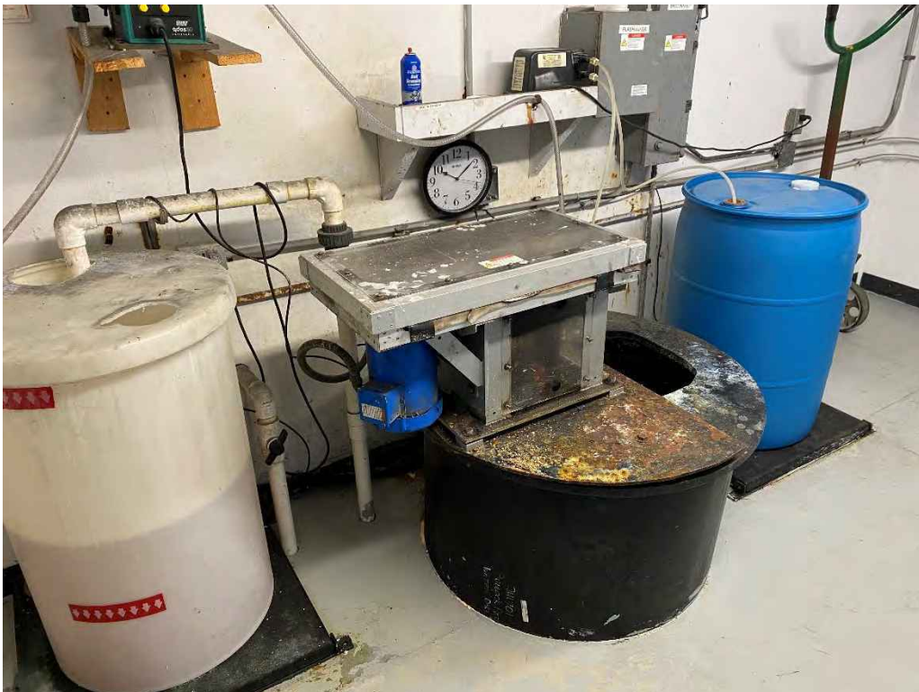
Upper Flash Mix and Polymer Feed System
