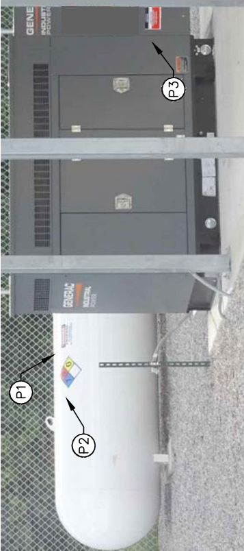
FIGURE 7 – PROPANE TANK & GENERATOR SIGNAGE
