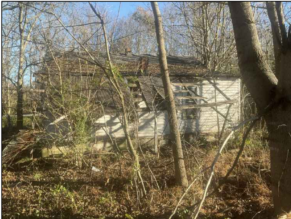
Photograph C-18: Collapsing house at site 15Gn88; facing southeast.
