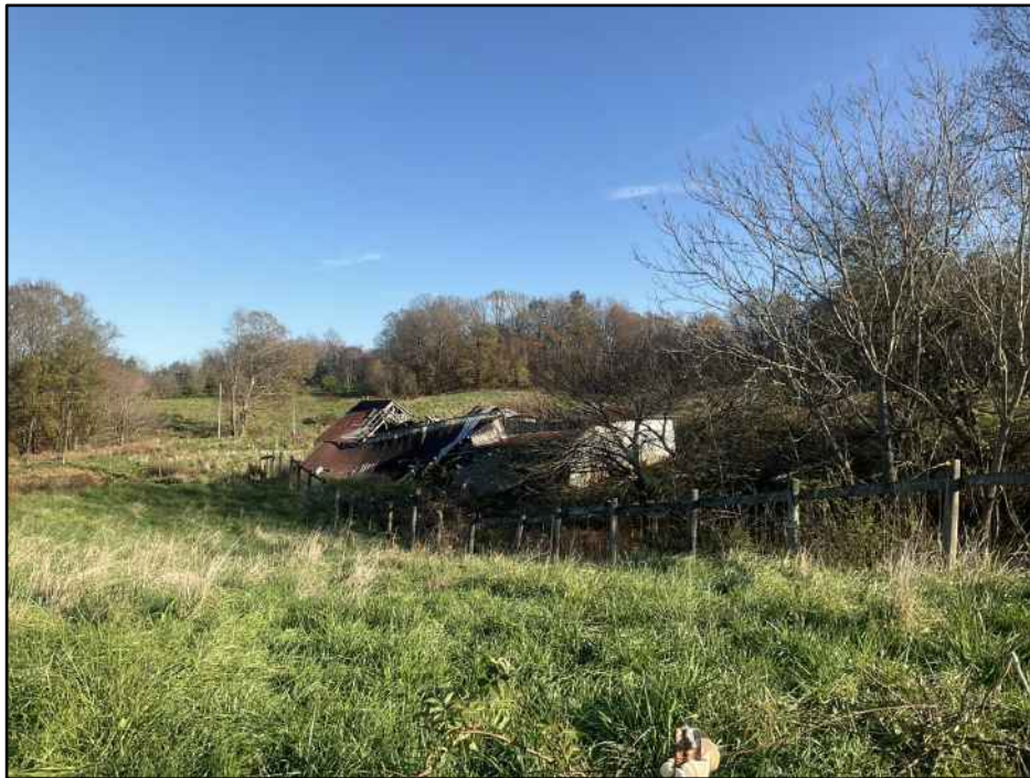
Photograph C-25: Collapsed structure at site 15Gn91; facing southeast.
