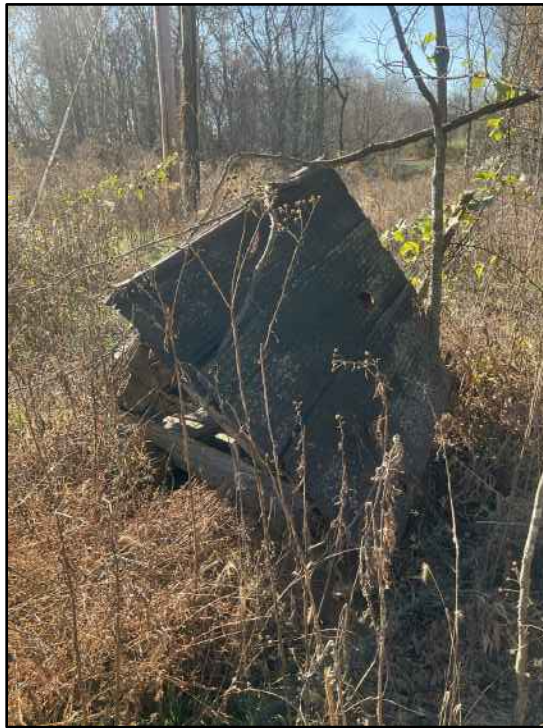
Photograph C-20: Collapsed outbuilding at site 15Gn90; facing west.
