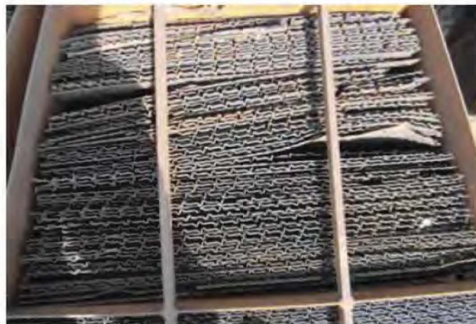
Figure 2-8 Air Preheater Heating Element Failure
