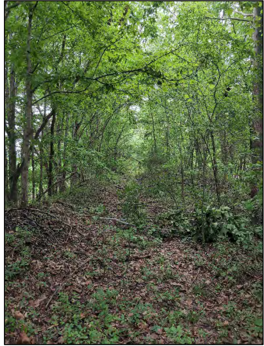
Abandoned railroad bed above culvert
