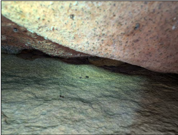
Bat guano found in the wall of the culvert
