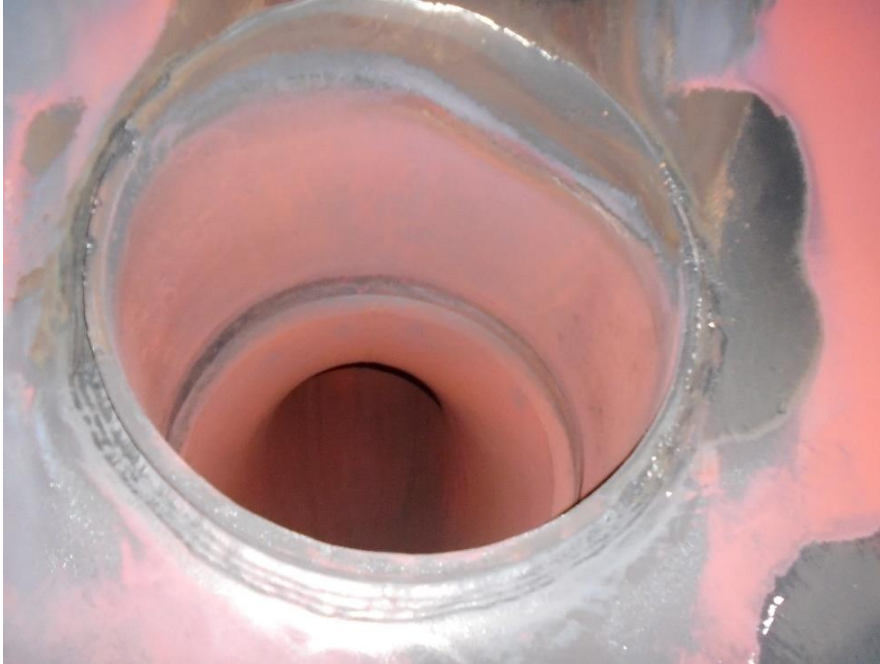
Steam inlet erosion.
