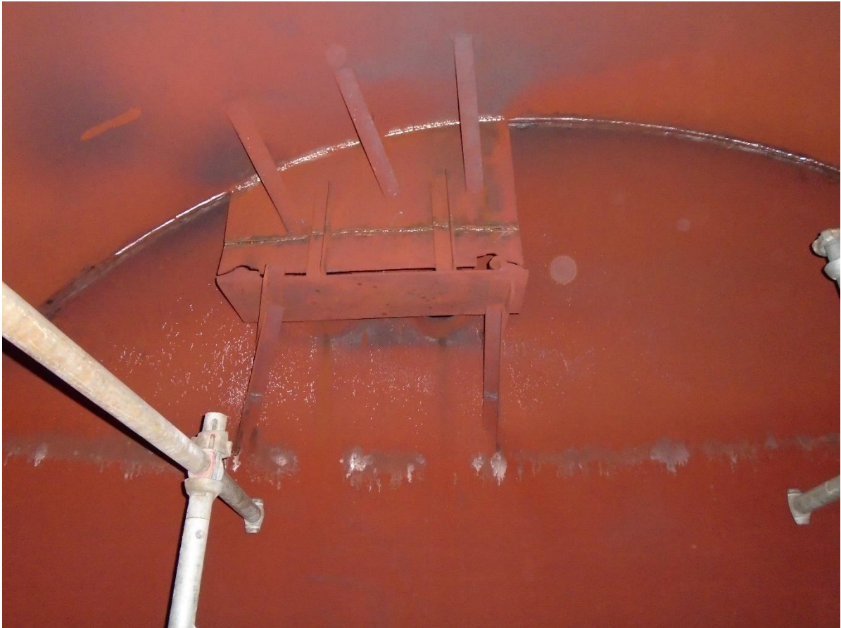
Cracked baffle plate in storage tank.
