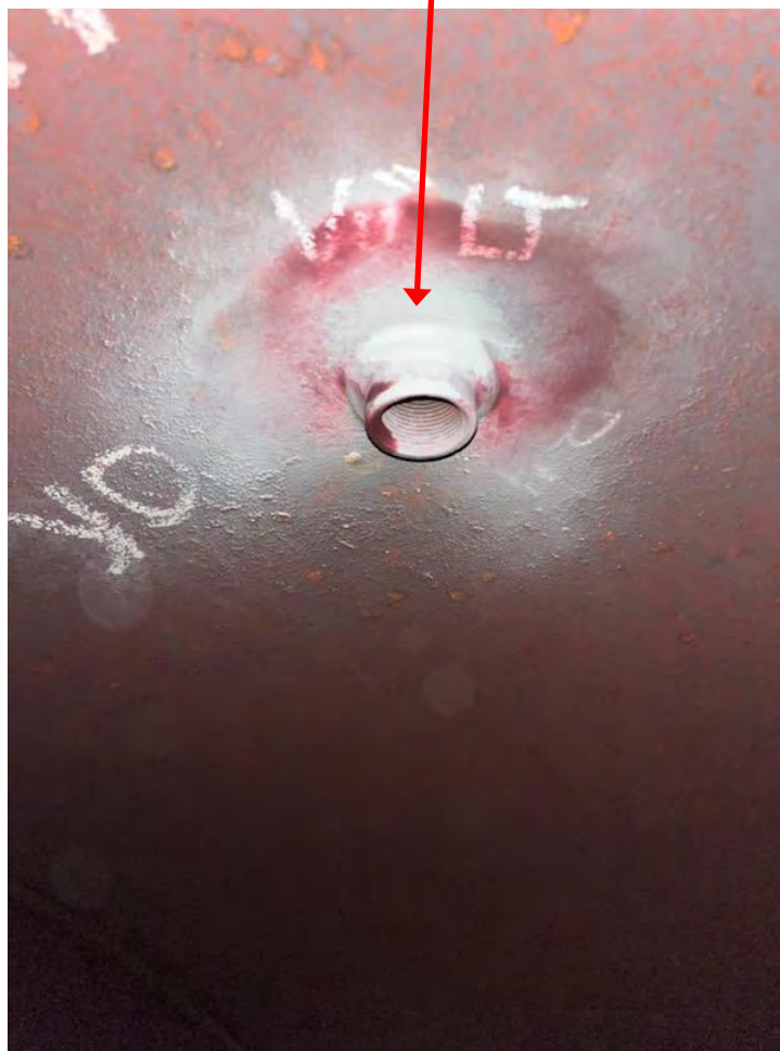
Fig. 61. Photographs of the indication at penetration No. P-4 on the deaerator storage tank.
