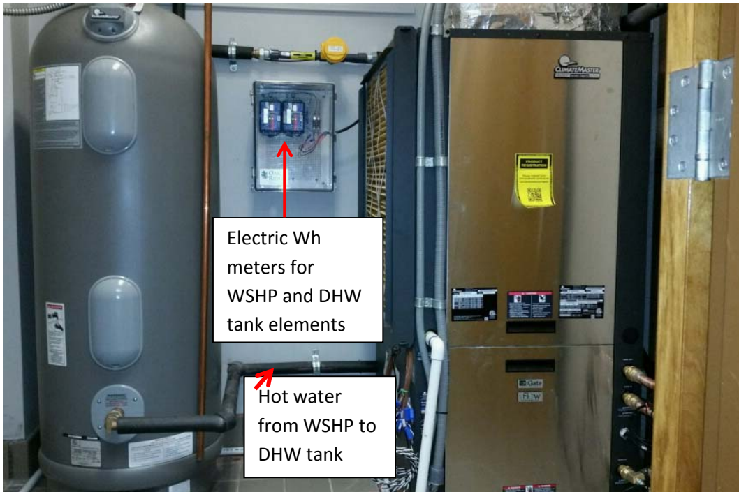
Figure 4. Trilogi WSHP system as installed at the Knoxville, TN test site
