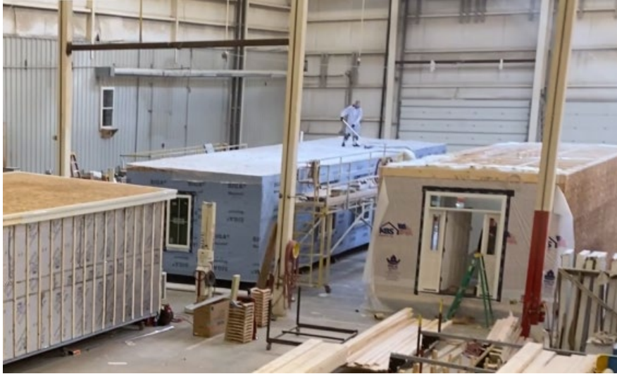
Figure A16. Bay 15 on the left - Touch-up, Exterior Wrap, Ship-Loose, and Labels.
