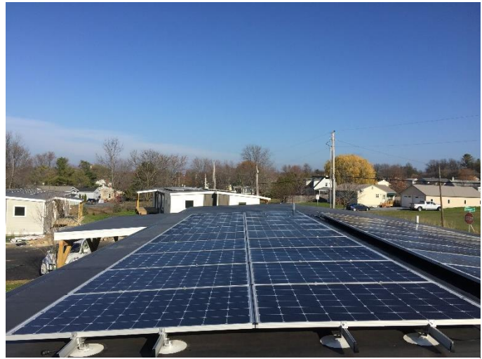
Figure 6: Solar PV system on a flat roof.
