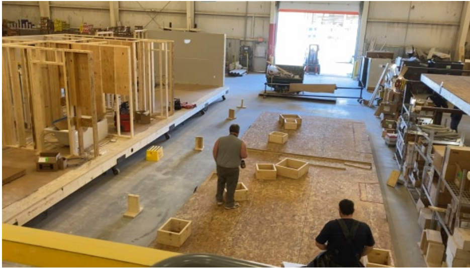
Figure A4. Bay 3 - Exterior and Mate Wall Set
