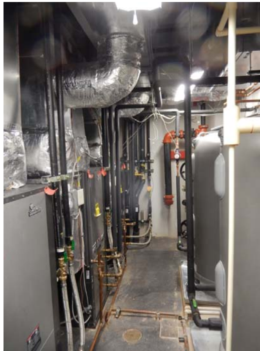
Figure 9. Oklahoma City host building mechanical room; instrumented Trilogy is on lh side against back wall; Trilogy HW tanks at right (Source: ClimateMaster)
