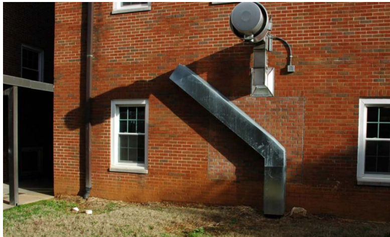
Figure 12. GHX loop headers attached to wall outside kitchen facility, Knoxville site
