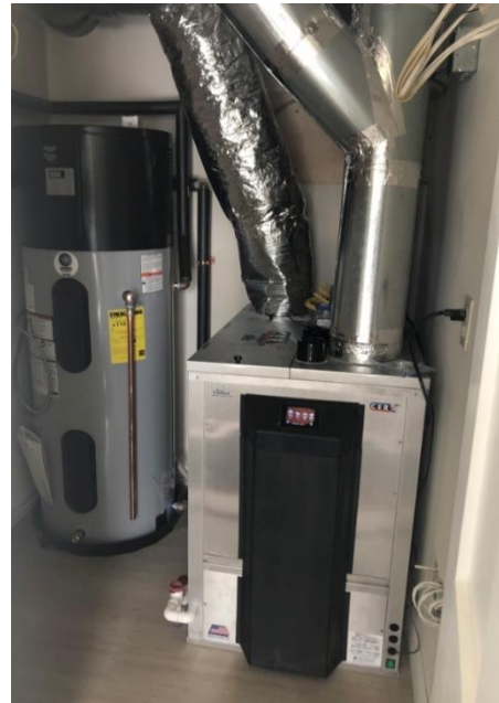
Figure 16: CERV and heat pump water heater in mechanical closet.
