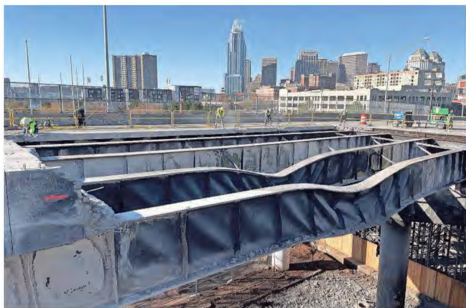
Officials are aiming to complete three years of work in five months on the Daniel Carter Beard Bridge after a Nov. 1 fire that warped steel beams and concrete decks. PHOTOS PROVIDED BY OHIO DEPARTMENT OF TRANSPORTATION
