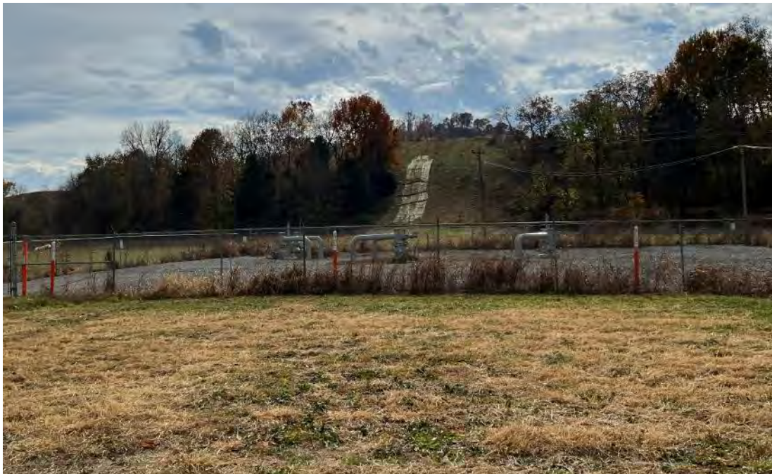
Figure 6-24: Liberty Natural Gas Metering Station
