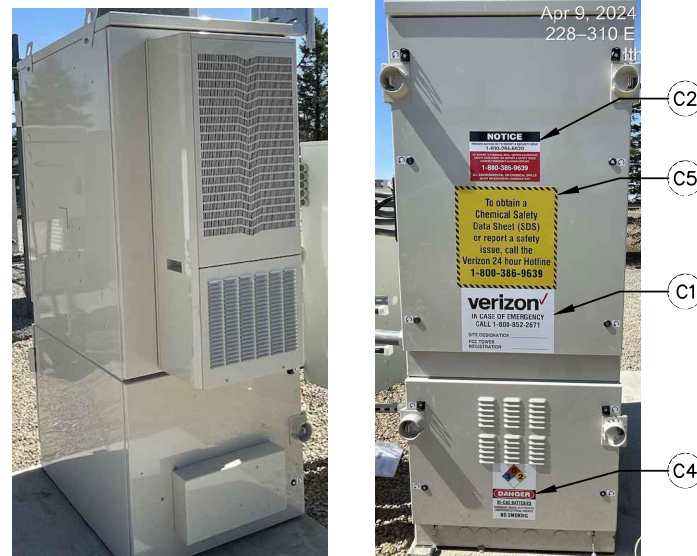
FRONT REAR FIGURE 1 - EQUIPMENT CABINET SIGNAGE
