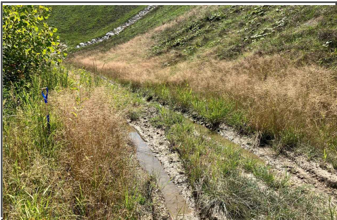
Photograph 6: View of Wetland 3, located in a low spot along an access road upslope of Wetland 1. August 12, 2024.
