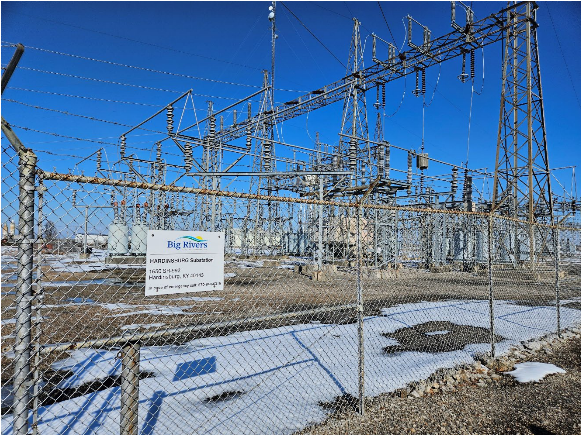
Figure C-17. Big Rivers Substation
