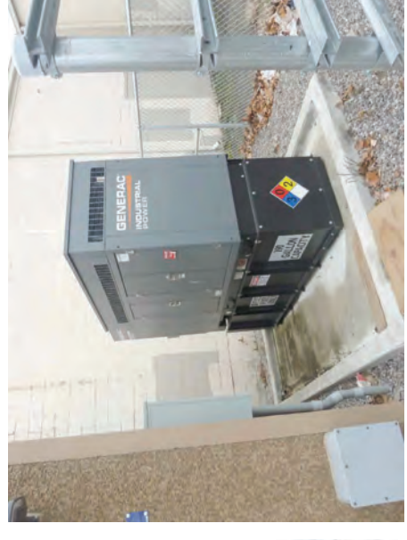
FIGURE 6 - DIESEL GENERATOR SIGNAGE
