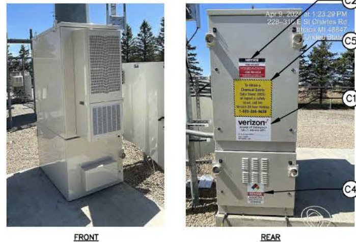
FIGURE 1 - EQUIPMENT CABINET SIGNAGE
