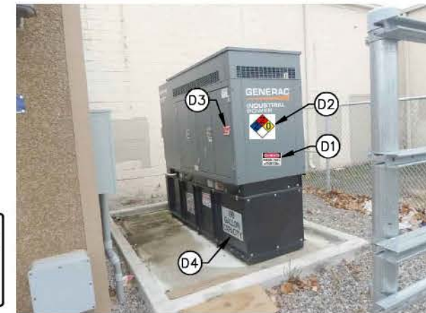
FIGURE 6 - DIESEL GENERATOR SIGNAGE
