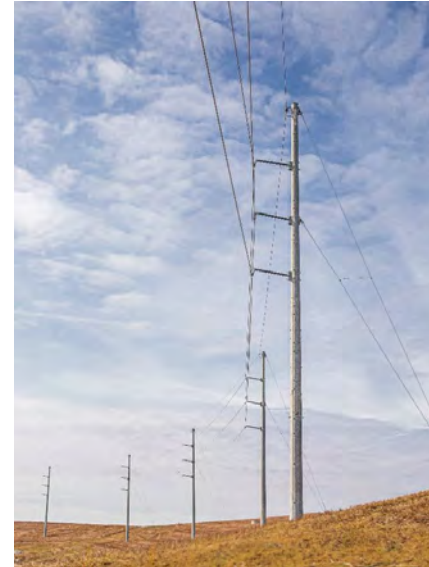
*Example of steel transmission poles – final design to be determined
