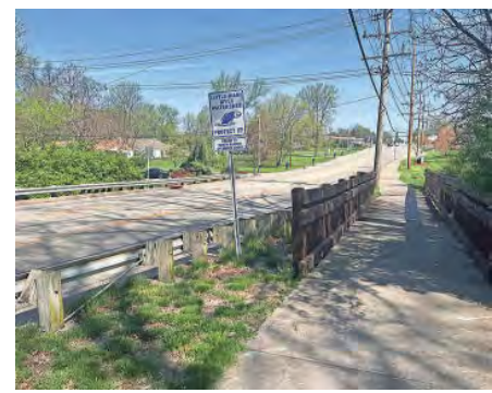
The Kenwood Road bridge will be under construction for more than two months as crews work to reconstruct failing infrastructure and rebuild a pedestrian bridge. CITY OF BLUE ASH
