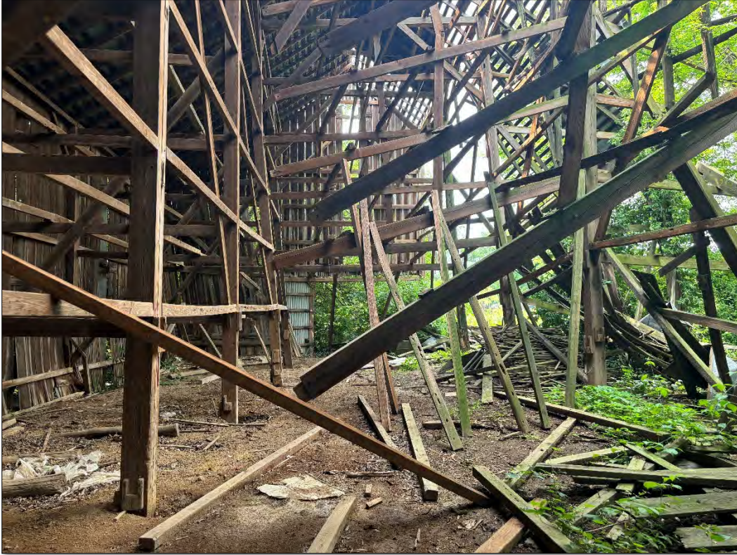
Photograph 11. Dilapidated barn in south-central portion of subject property
