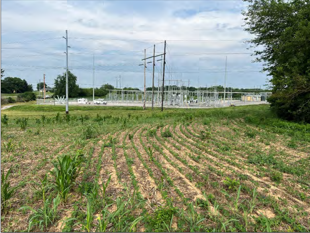
Photograph 9. View of EKPC's Avon substation
