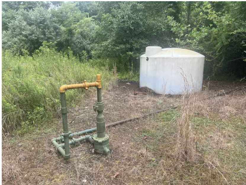
View of the oil/gas well and AST with significant staining and stressed vegetation along the western portion of the Subject Property
