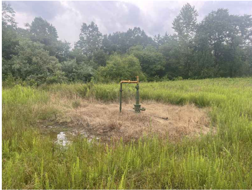
View of the stressed vegetation observed surrounding a wellhead along the western portion of the Subject Property
