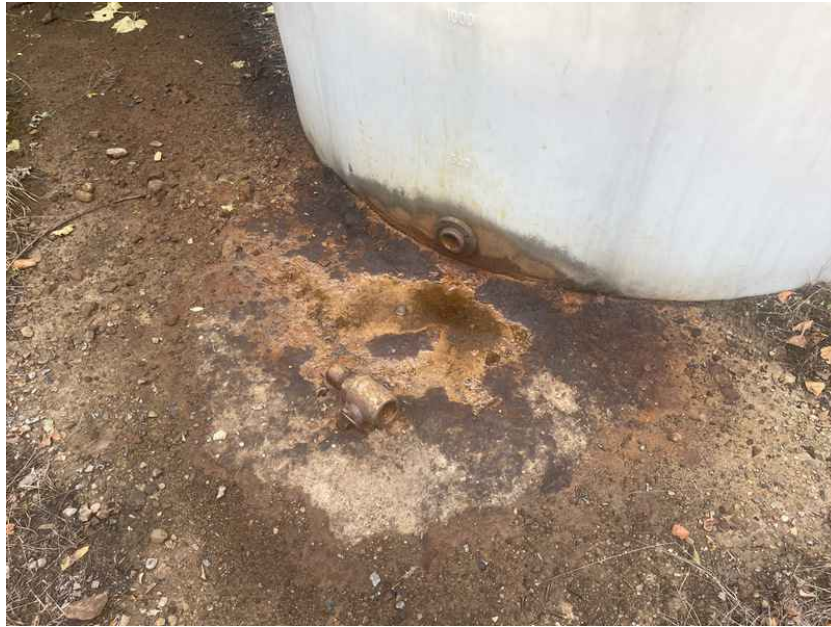
View of the significant staining beneath the AST
