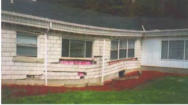
Figure 4: Typical cracking of walls/foundation due to Trough Subsidence (Duquesne Energy Initiative 2020)
