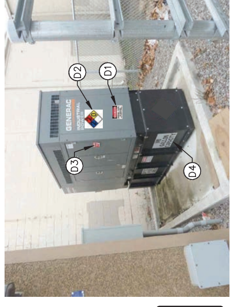
FIGURE 6 - DIESEL GENERATOR SIGNAGE
