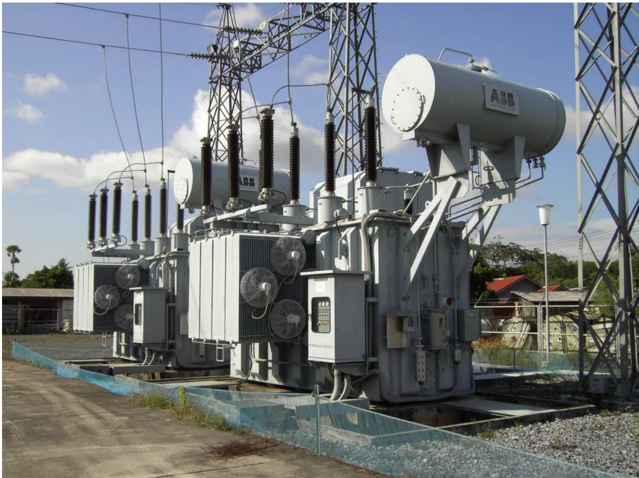
Picture (6) Substation Transformer 6
