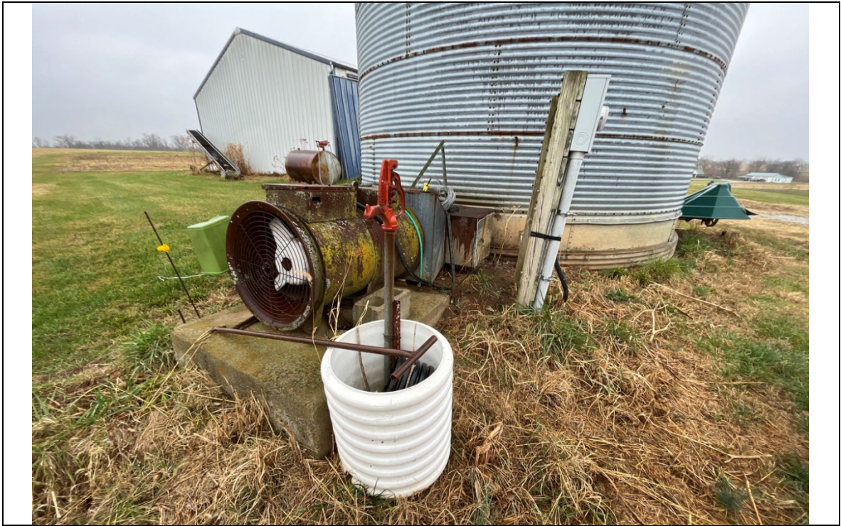
Photograph: 17 | View of a pump connected to a silo.
