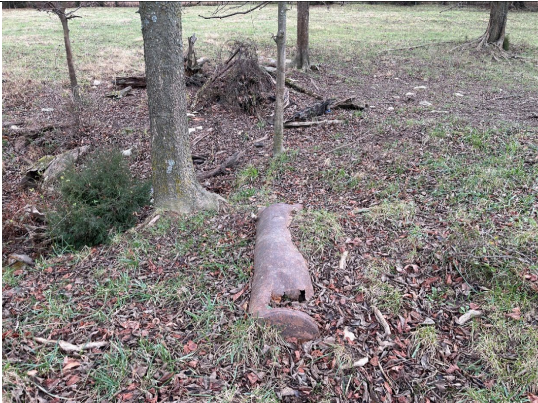
Photograph: 13 View of the punctured tank located within the northern portion of the Site.
