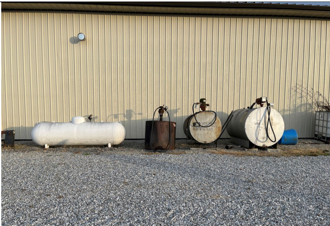
Photograph: 14 View of ASTs land tote located within the eastern-central portion of the Site.
