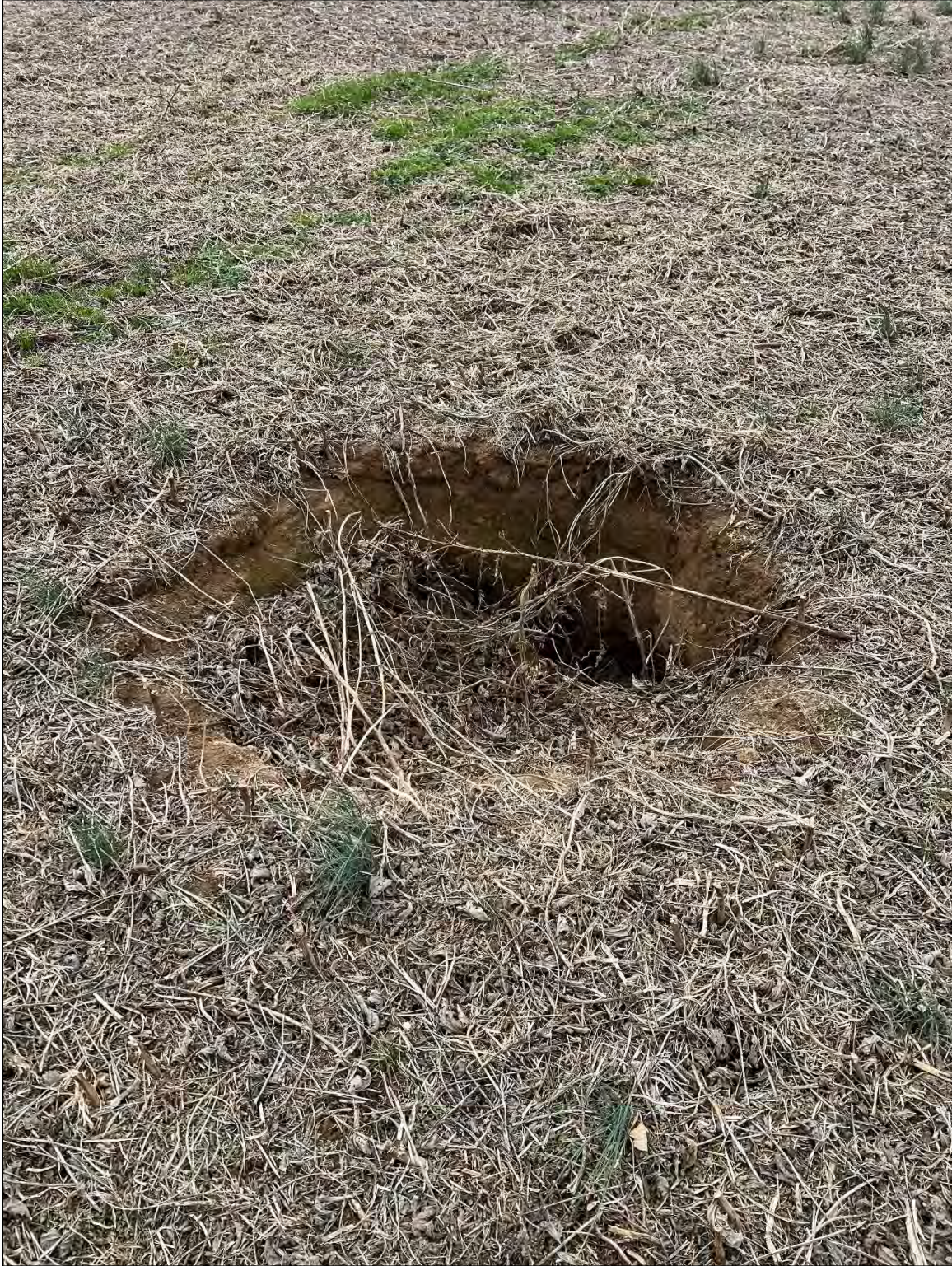
G2 observed depression No. 10 of 11 Approximately 90 feet North and 400 feet West from test pit T-29 Latitude 37.62480° N Longitude 85.27308° W
