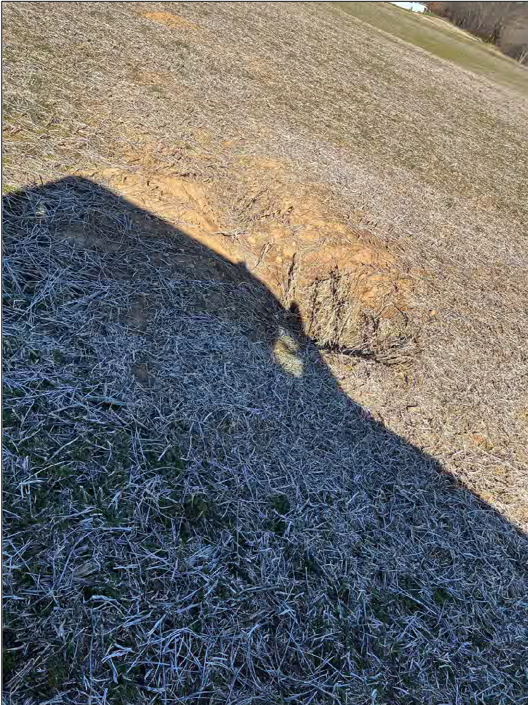
G2 observed depression 5 of 11 Approximately 50 feet South and 200 feet West from test pit location PD-07 Latitude: 37.650278 N Longitude: 85.272222 W
