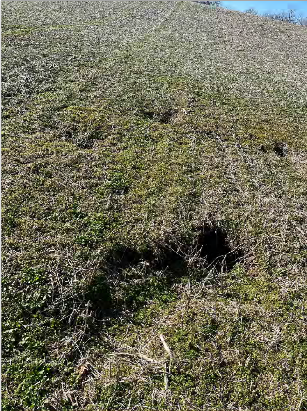
G2 observed depression 4 of 11 Approximately 50 feet North and 100 feet West from soil boring location PD-07 Latitude: 37.650556 N Longitude: 85.271667 W
