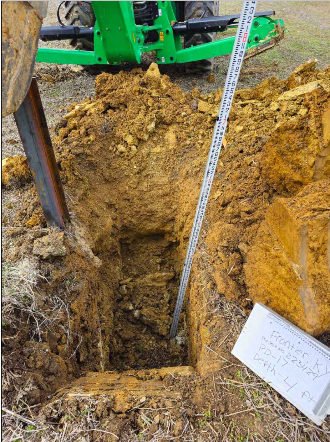
Test Pit ID: PD-17 Test Pit Depth: 4 feet Date: December 16, 2023 Field Engineers: Mohamad Majed Timothy Dehayes
