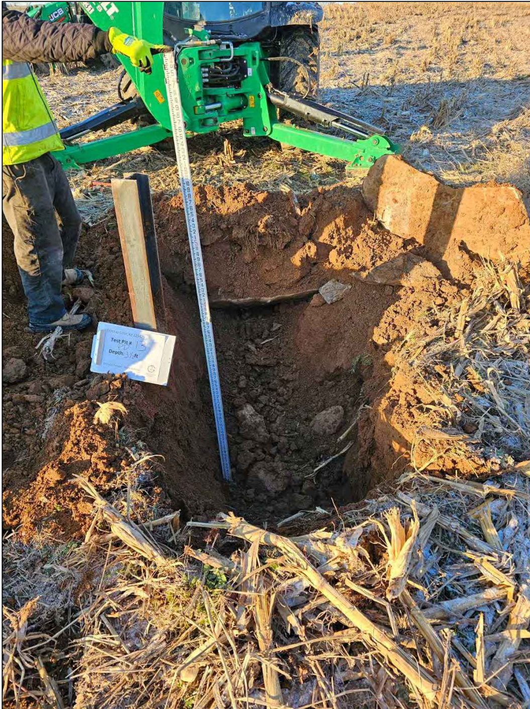
Test Pit ID: PD-13 Test Pit Depth: 3-1/2 feet Date: December 19, 2023 Field Engineers: Mohamad Majed Timothy Dehayes
