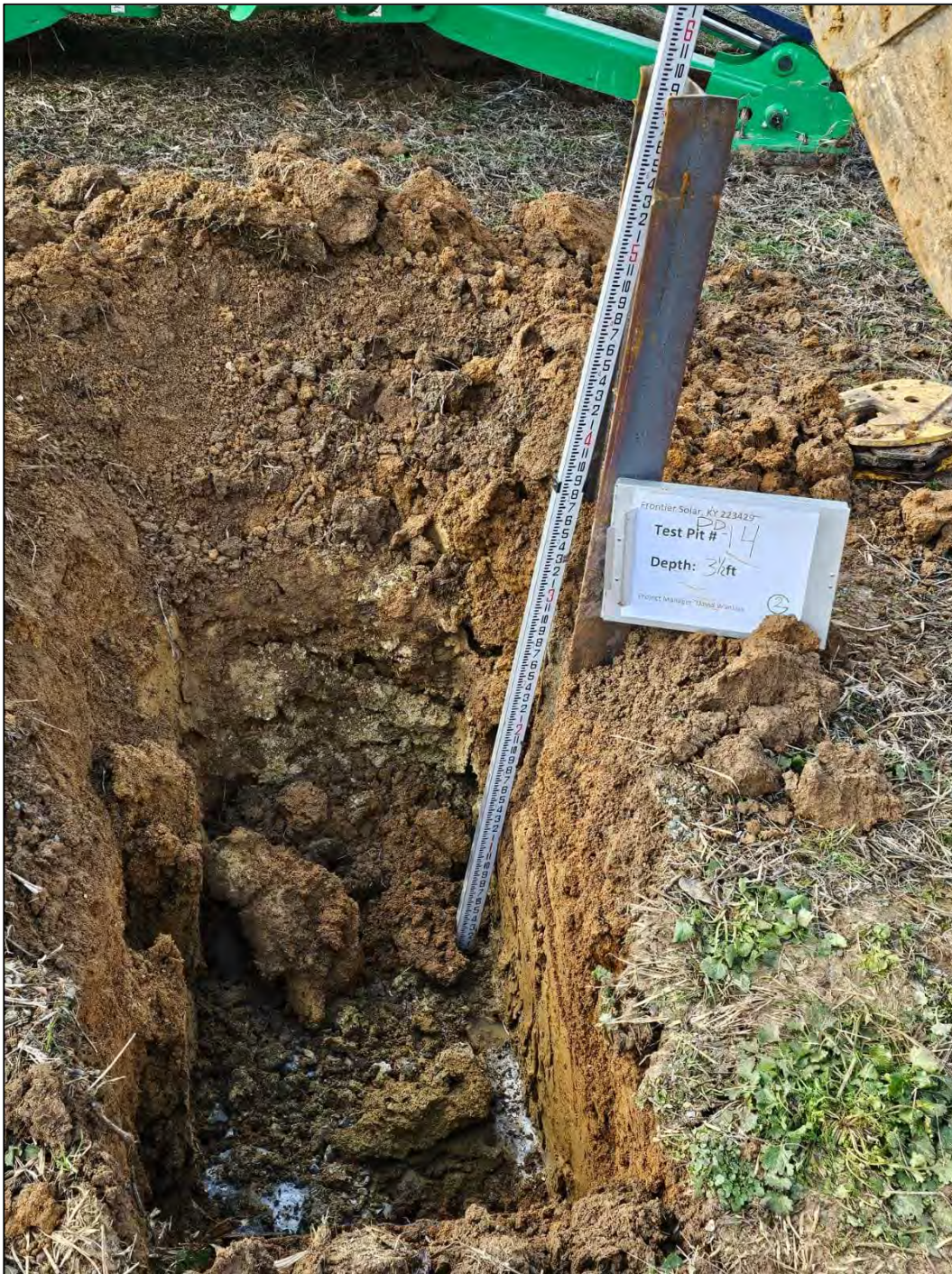
Test Pit ID: PD-14 Test Pit Depth: 3-1/2 feet Date: December 18, 2023 Field Engineers: Mohamad Majed Timothy Dehayes
