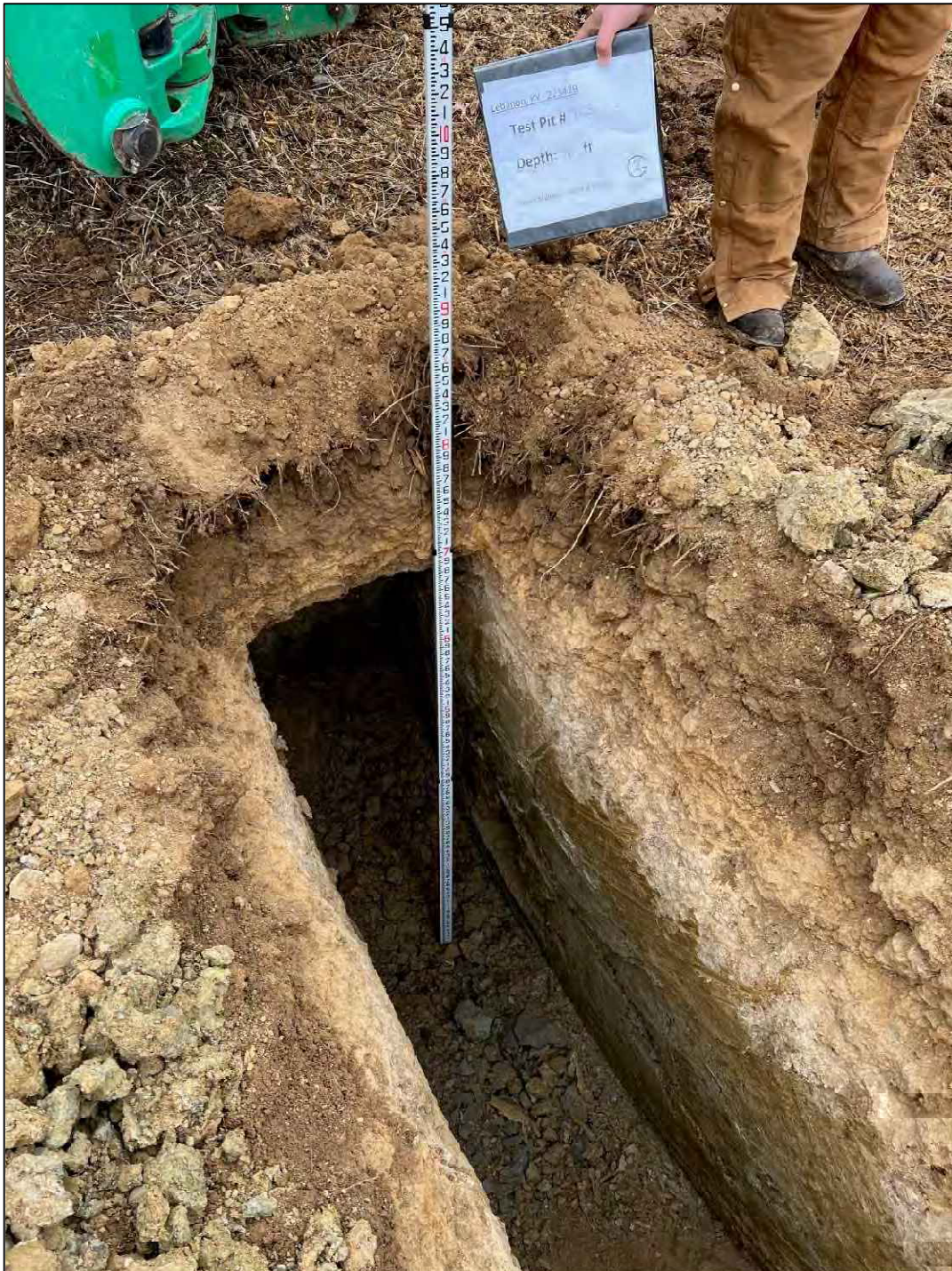
Test Pit ID: T-03 Test Pit Depth: 9 feet Date: November 15, 2022 Field Engineer(s): Zachery Lilly Steve Misze
