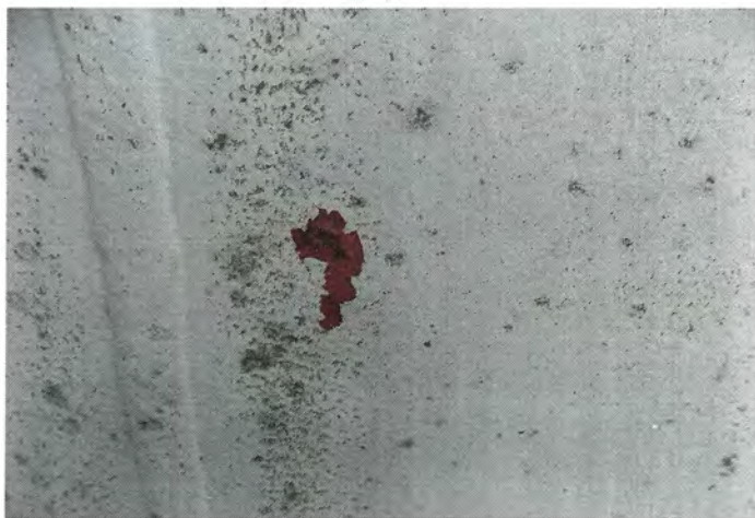
Photo shows an area of delamination along the lower riser where the red primer can be seen.
