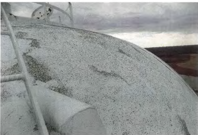
Photo shows mildew staining along the northwest upper knuckle.
