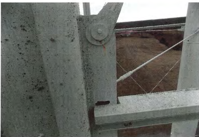
Photo shows a small area of corrosion present at the pinned windage rod connection.
