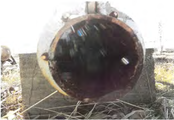
Photo shows the overflow discharge. A fine mesh insect screen should be installed between the pipe flanges.
