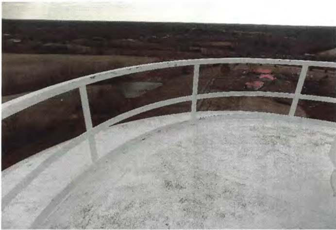
Photo shows the southeast section of the roof and 42" tall roof handrail. Mildew covers the surfaces.
