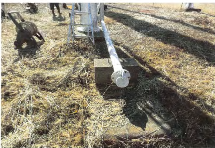
Photo shows the overflow pipe's discharge point and concrete splash pad. The overflow is equipped with a flapper valve.
