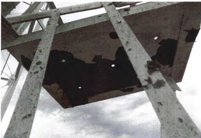
Photo shows delamination and corrosion present on the underside of a ladder platform.
