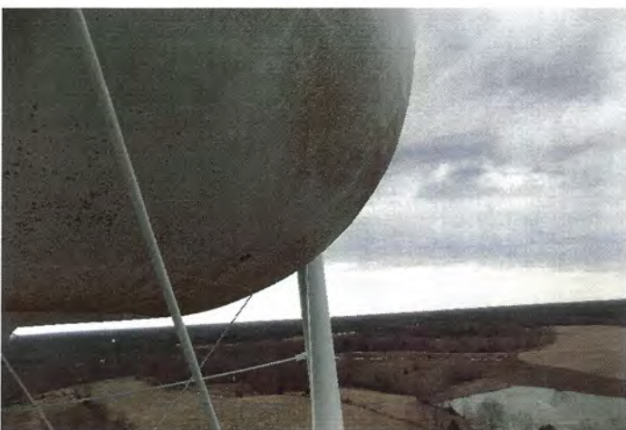
Photo shows mildew present on the west section of the lower knuckle.
