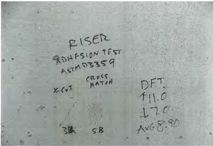
Photo shows the results of adhesion tests performed per ASTM D3359 along the lower riser. The adhesion test results are a 3A and a 5B. The Dry Film Thickness (DFT) in the test area ranged from 7.0-11.0 mils and averaged 8.90 mils. The tank is a candidate for an overcoat.
