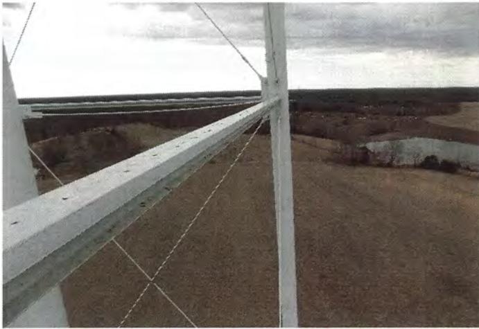
Photo shows the west facing upper strut. The existing coating system in this area is nearing the end of its life cycle.
