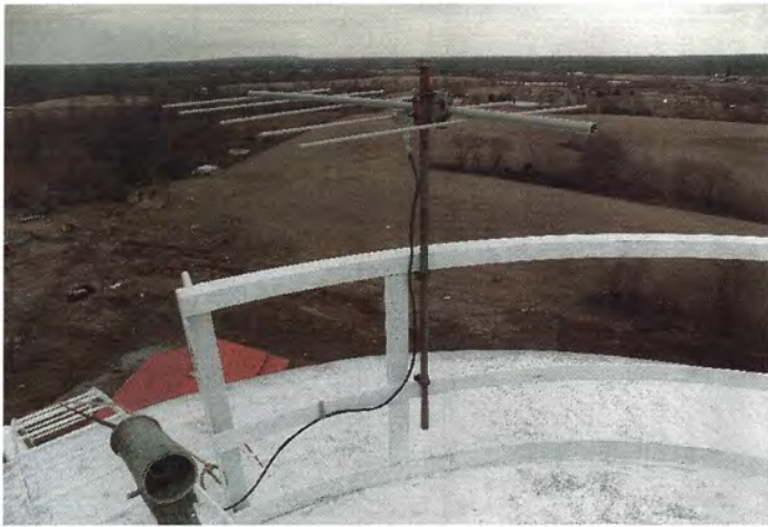
Photo shows an antennae affixed to the roof corral.
