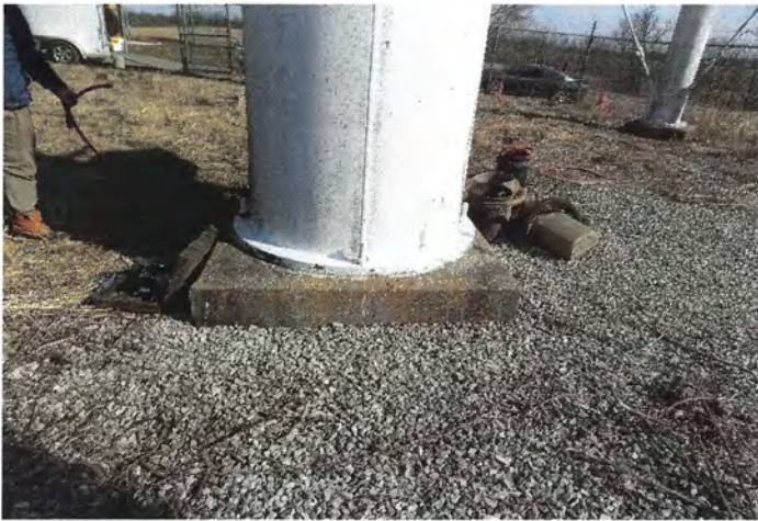
Photo shows the riser base, anchor bolts, and concrete foundation.
