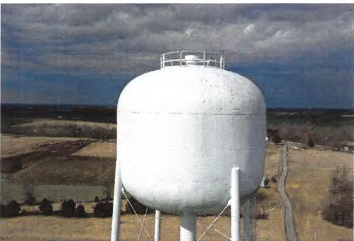
Photo shows the east section of the shell. The existing coating system has lost its gloss.
