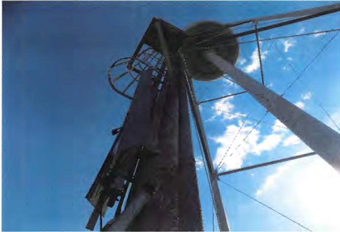
Photo shows the aluminum climb prevention shield. The shield is damaged and should be replaced.
