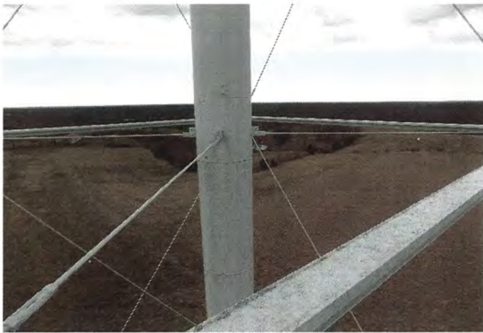
Photo shows the existing coating system on the middle section of the riser continues to protect the steel substrate.
