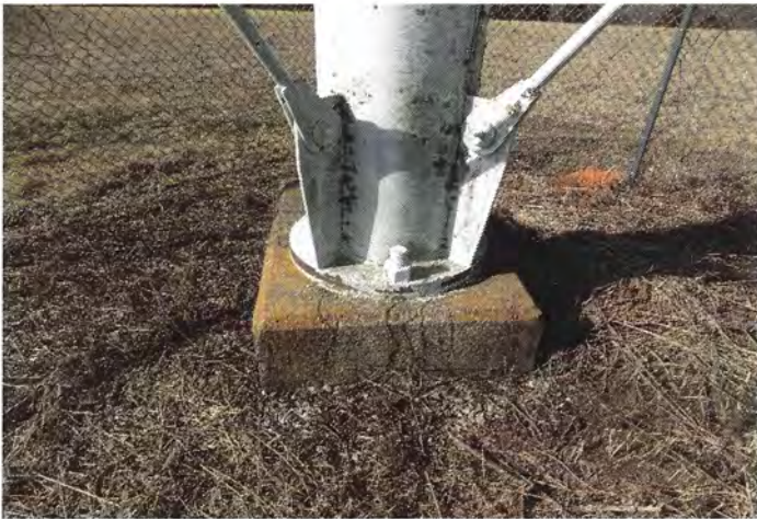
Photo shows the leg base plate, anchor bolts, and concrete foundation. The anchor bolts are in good condition. The uncoated concrete is in sound condition.
