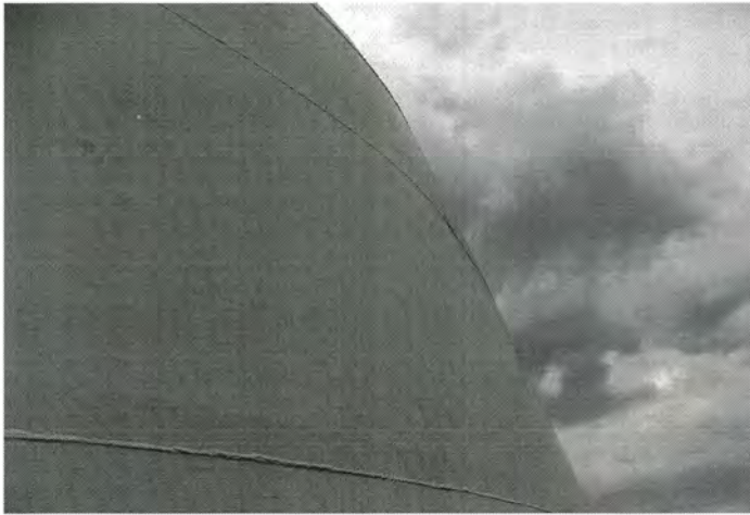
Photo shows the west section of the shell. The existing coating system continues to protect the steel substrate.
