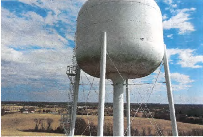
Photo shows the south section of the shell and lower knuckle. The existing coating system is close to the end of its life cycle.
