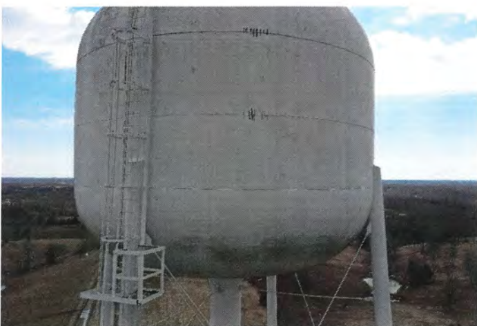
Photo shows the west section of the shell. The finish coat has become chalky and dull.
