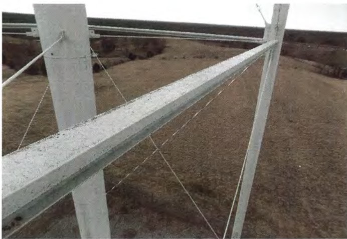
Photo shows the west facing lower strut. The topcoat in this area has become chalky and dull.
