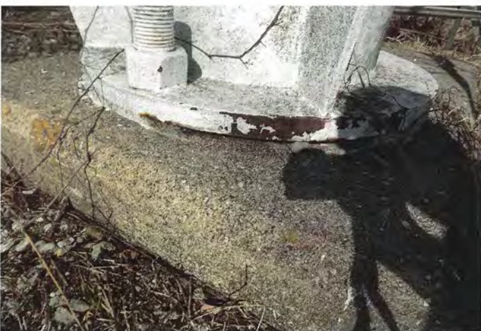
Photo shows an area of grout missing along the northwest leg to foundation connection.
