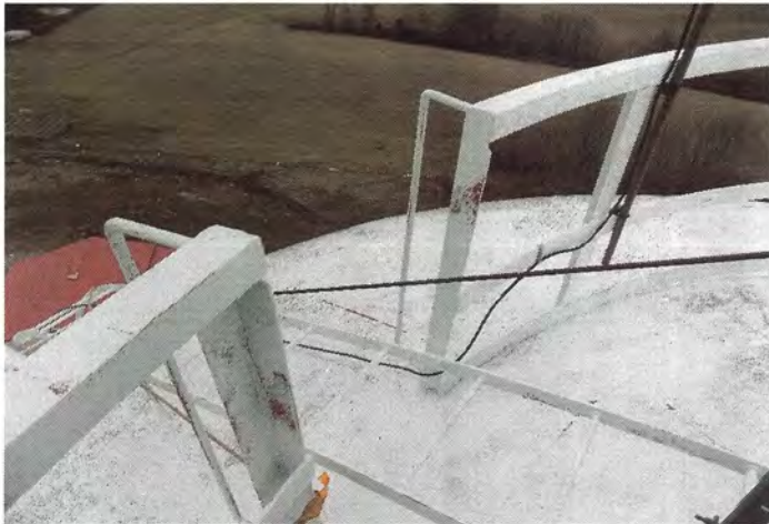
Photo shows the roof handrail opening and grab bars. Safety chains or a swing gate should be installed across the opening.
