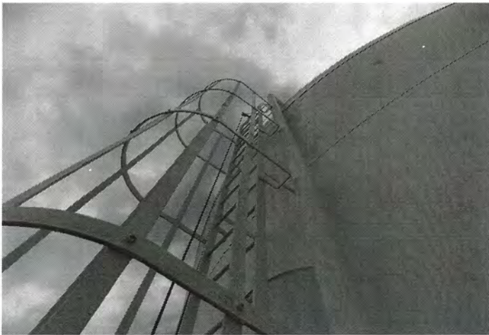
Photo shows the upper section of the tank ladder and overflow pipe on the northwest section of the shell. The cage is not required since the ladder is equipped with a fall prevention cable. The cage could be removed.
