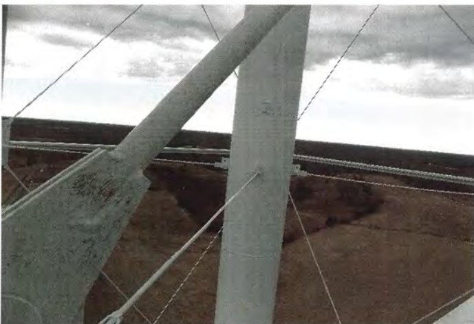
Photo shows the existing coating system on the upper section of the riser continues to protect the steel substrate.
