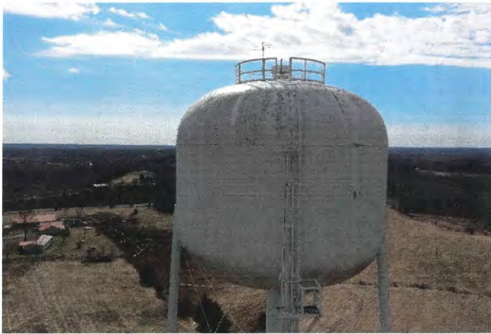
Photo shows the northwest section of the shell and ladder. The existing coating system continues to protect the steel substrate.
