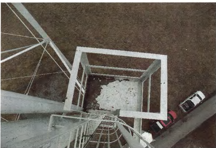
Photo shows corrosion present on the ladder platform floor.
