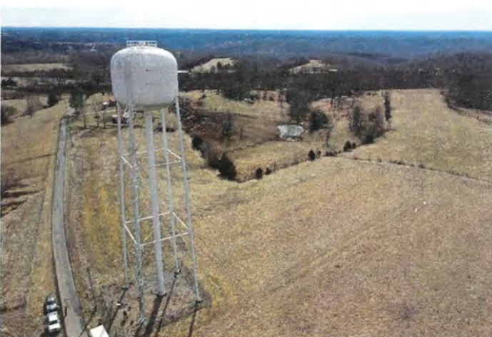
Photo shows an overall view of the west side of the tank. The tank has two struts and three panels.
