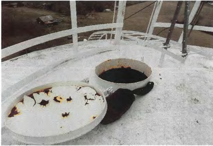
Photo shows the 24" diameter roof access hatch with hinged cover. Corrosion is present along the frame and hatch cover. The coating on the inside of the cover is extremely brittle.
