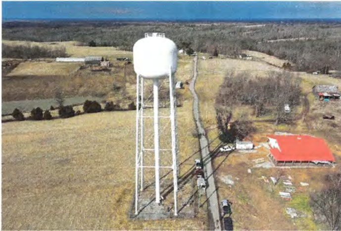
Photo shows an overall view of the east side of the tank and tank site.
