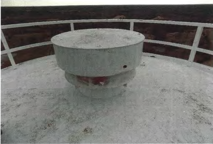
Photo shows the 24" diameter roof vent with a steel cover.
