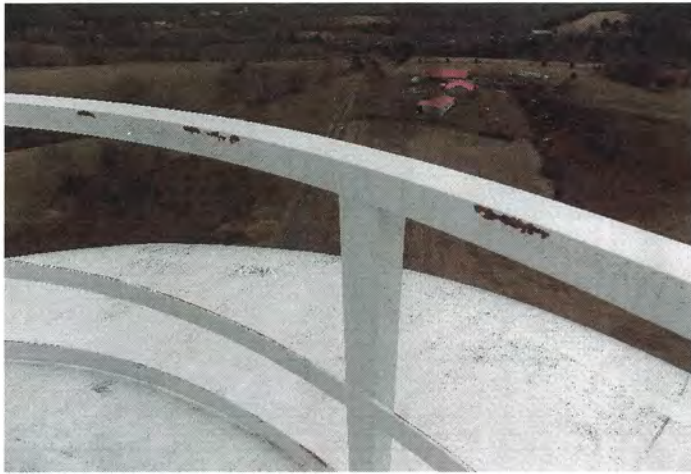
Photo shows areas of corrosion present along the roof corral railing.
