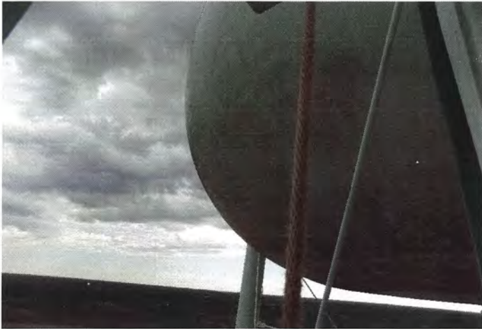
Photo shows the north lower knuckle. The existing coating system in this area has lost its gloss.
