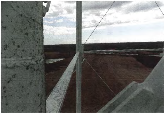
Photo shows mildew present on the north facing lower strut.
