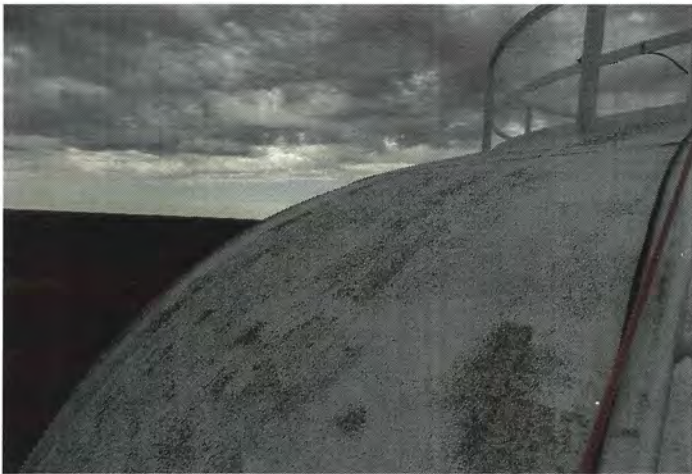
Photo shows heavy mildew present on the north section of the upper knuckle.
