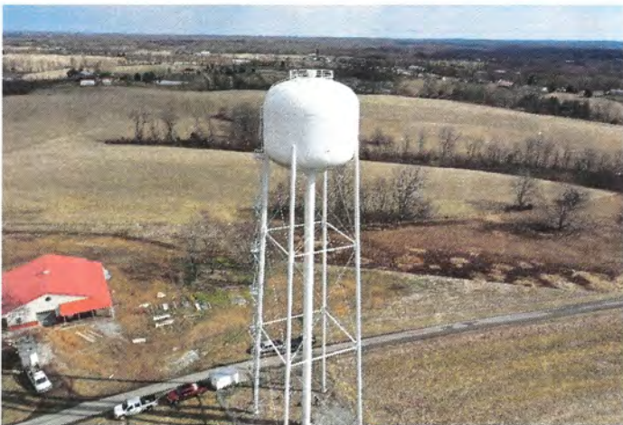
Photo shows the south side of the tank. The tank does not have an external balcony.
