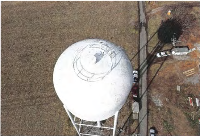
Photo shows an overall view of the roof. The roof is equipped with a 42" tall handrail.
