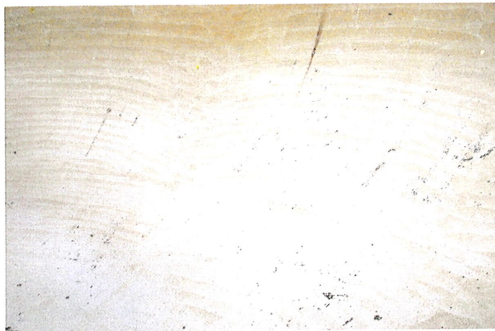
Photo shows the west section of the lower knuckle after cleaning. Delamination to the steel and between coats is visible.
