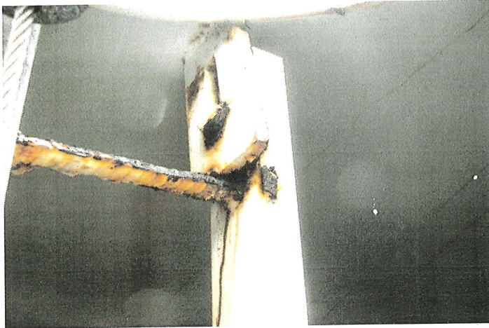
Photo shows the other ladder to roof connection point. Stainless steel hardware should be installed at this connection as well.
