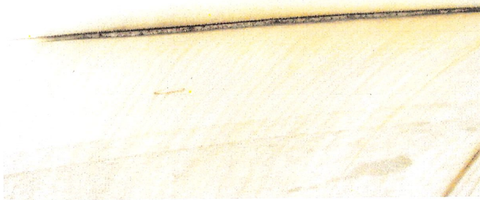
Photo shows a roof lap seam. All roof lap seams should be sealed with a flexible caulking compound.
