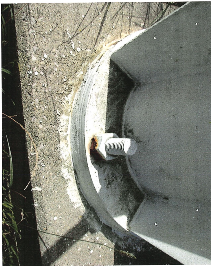
Photo shows the 1.75" column anchor bolts. Each leg has 2 anchor bolts. Minor rust is visible along the nut to column flange interface.
