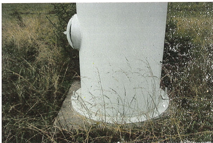
Photo shows the lower section of the riser and exposed concrete foundation. The concrete is in sound condition.
