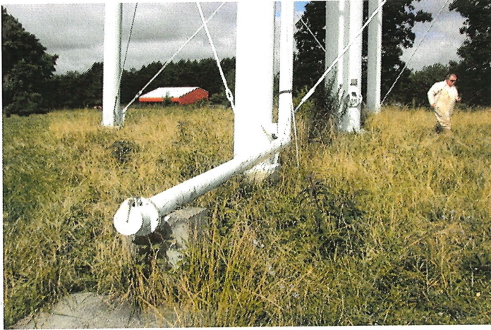
Photo shows the lower section of the 6" overflow pipe along the southeast leg.
