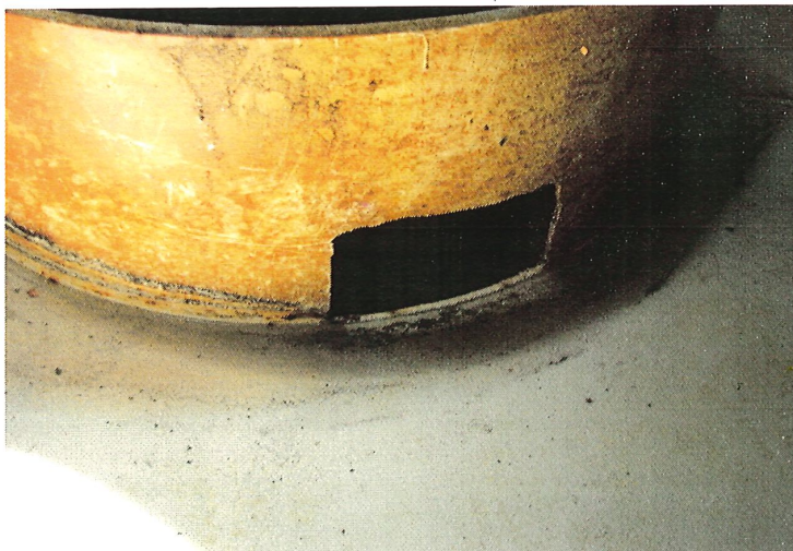
Photo shows the riser mud drum and drain hole.
