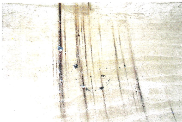
Photo shows an area of active corrosion cells and pitting present along the southwest section of the lower knuckle.
