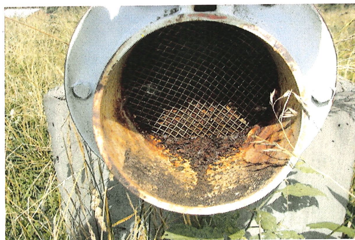
Photo shows the overflow pipe insect screen. Loose rust and paint chips should be removed from the interior of the screen to prevent clogging.
