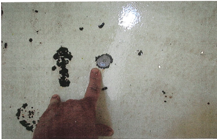
Photo shows a pit found along the south section of the lower knuckle. Some metal loss has occurred.
