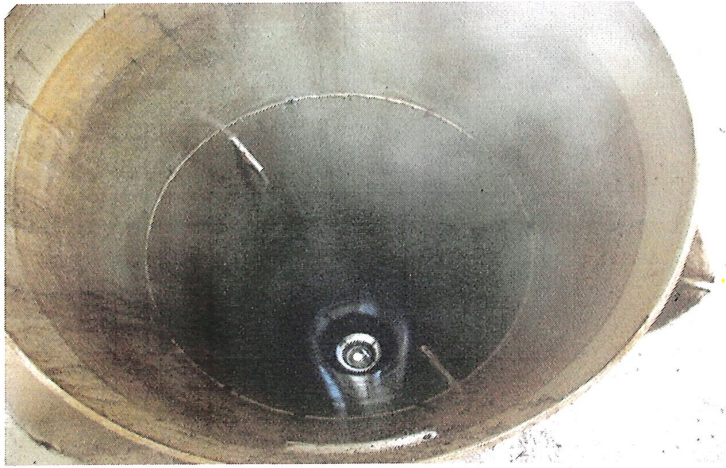
Photo shows the upper section of the riser. There is no ladder in present.
