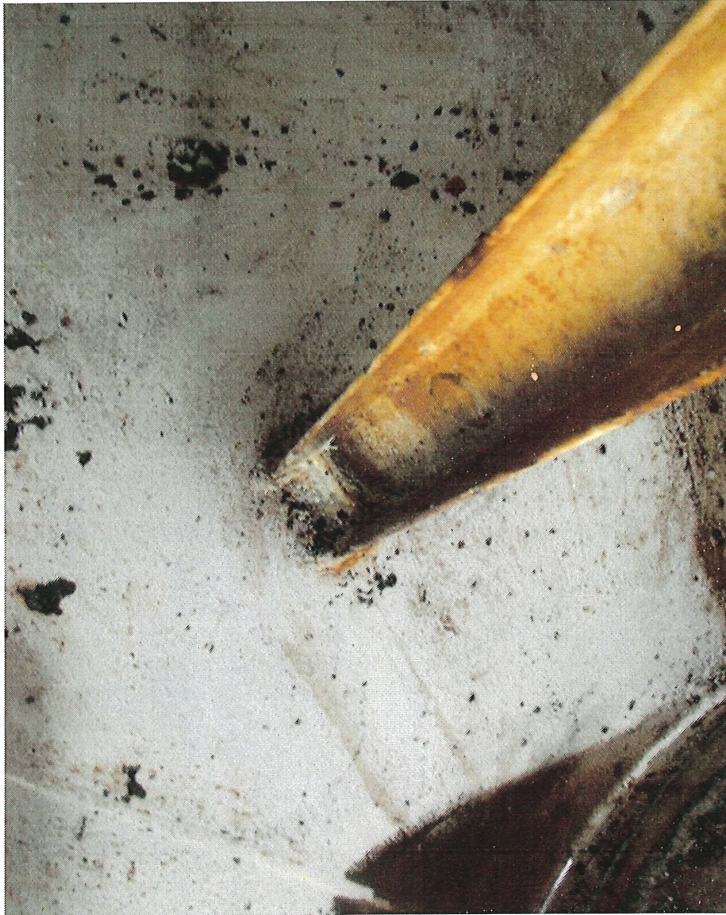
Photo shows the ladder to floor connection point. Delamination of the existing top coat can be seen in this area.
