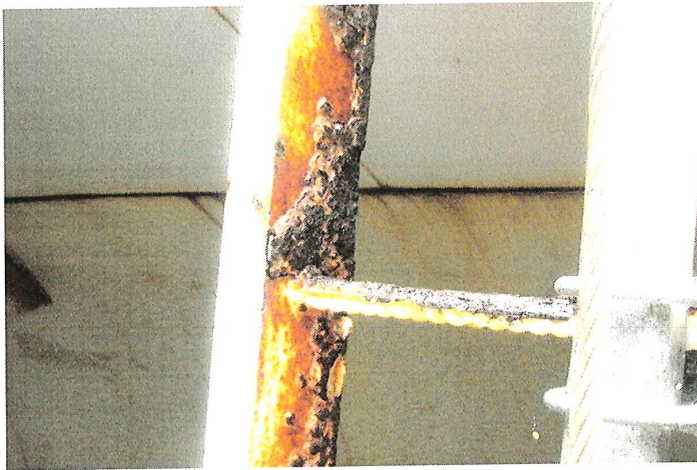
Photo shows heavy corrosion present along the upper section of the ladder rail and rungs.
