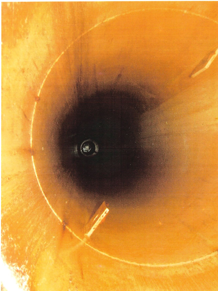
Photo shows heavy staining along the upper section of the riser. Active corrosion cells are visible along the weld seams.
