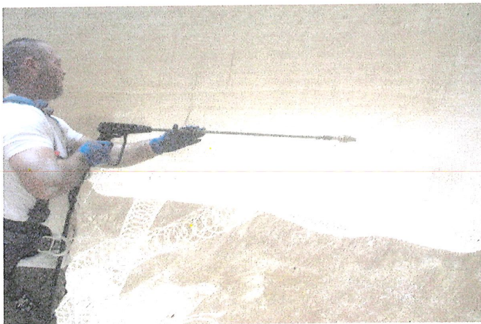
Photo shows a worker using a 4,000-psi pressure washer to remove staining along the lower knuckle. Contrast can be seen between cleaned and uncleaned areas.
