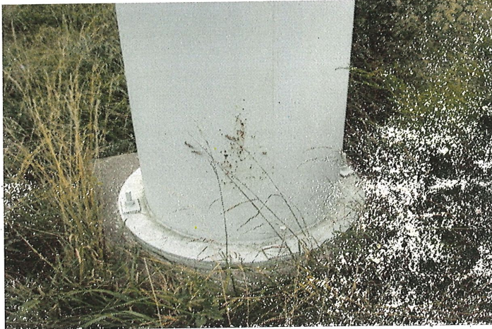
Photo shows active corrosion present along the lower section of the riser.
