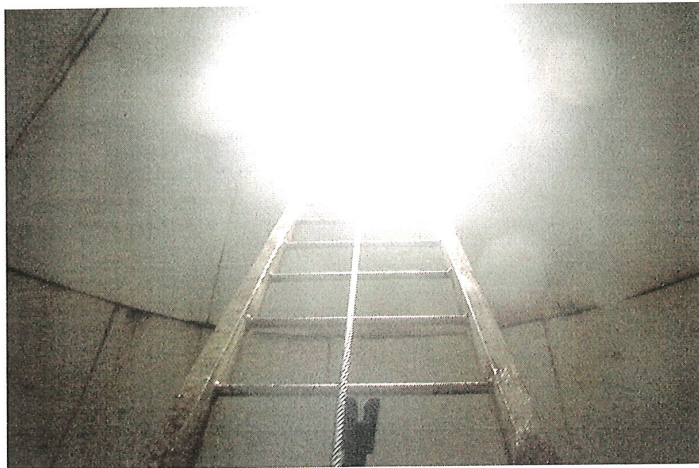
Photo shows the interior ladder equipped with a stainless steel cable style climber safety device that is in sound condition.
