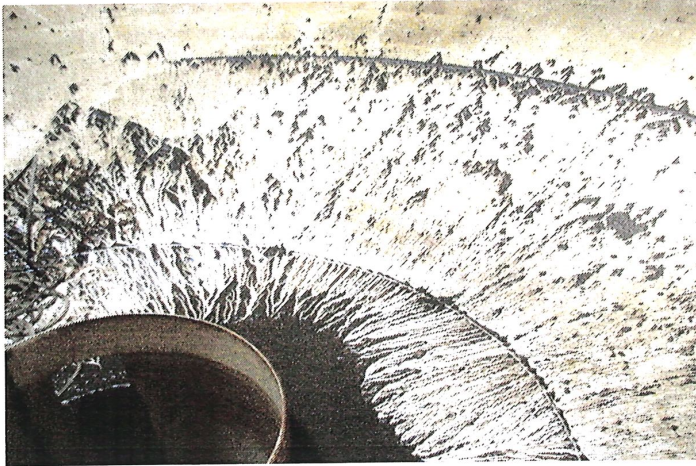
Photo shows sediment and staining present along the floor prior to high pressure water cleaning.
