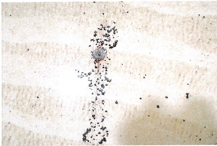
Photo shows an area of pitting along the east section of the lower knuckle.
