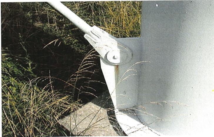
Photo shows minor rust bleed present along the northeast lower windage rod to leg connection point.
