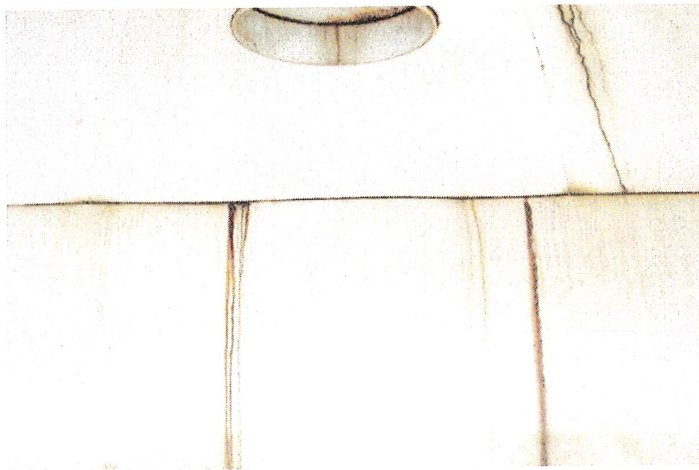
Photo shows active corrosion present along the northwest portion of the roof finger panels.
