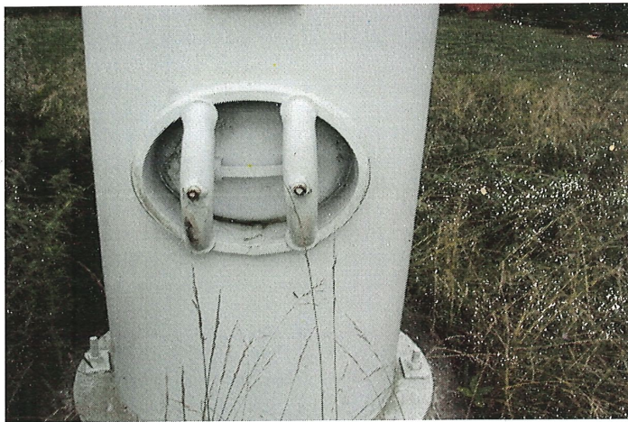
Photo shows the 18" oval riser manway. A new 30" bolted flanged riser manway with stainless steel bolts and brass nuts should be considered.
