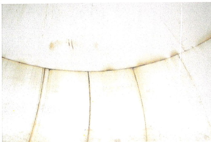
Photo shows the south section of the roof finger panels and upper knuckle. Rust bleed and staining is present throughout. All lapped seams should be sealed to prevent crevice corrosion.
