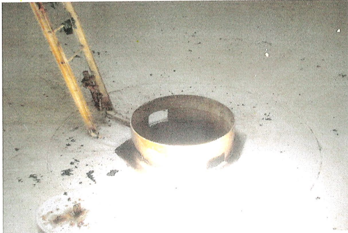
Photo shows the floor and riser opening after all sediment has been removed. A 42" handrail should be installed around the riser opening.
