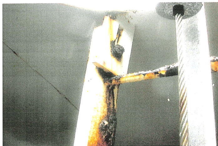
Photo shows the interior ladder to roof connection. New stainless steel bolts, washers, and nuts should be installed to replace the heavily corroded existing ones.
