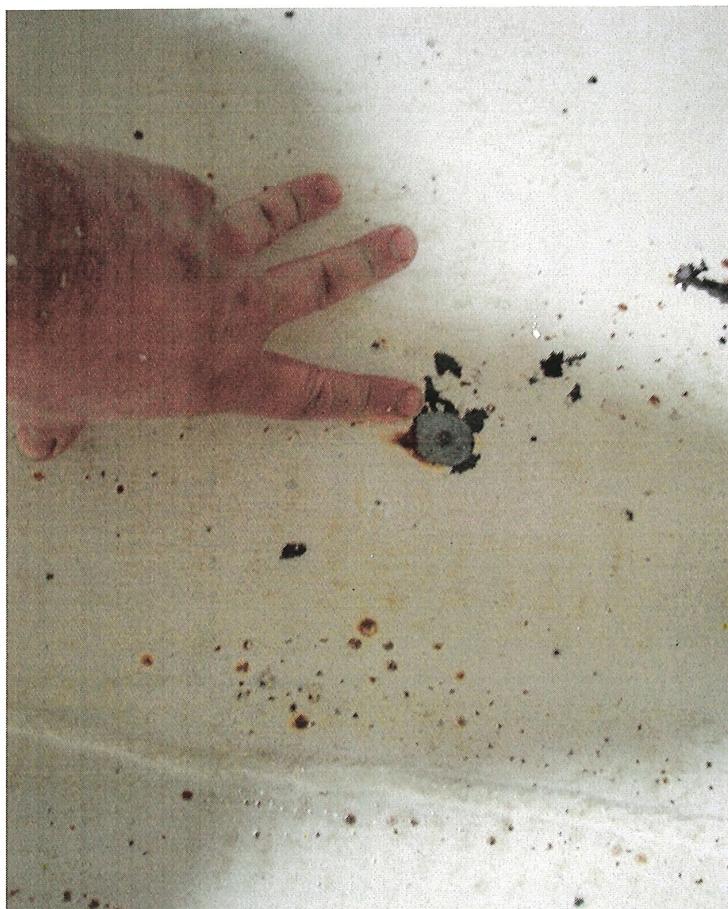
Photo shows metal loss occurring in another pit found along the south section of the floor.
