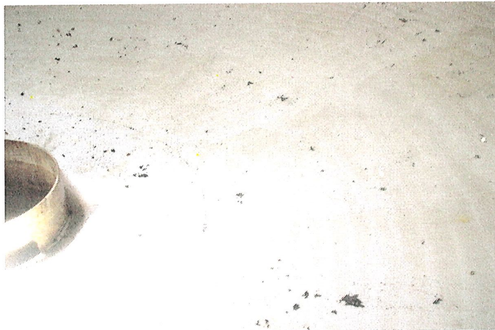
Photo shows the south section of the floor after high pressure water cleaning. Delamination of the top coat can be seen.
