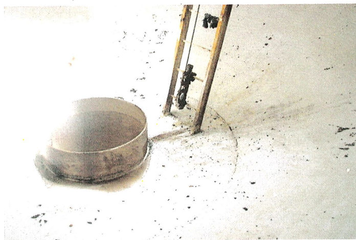
Photo shows another view of the floor after sediment removal. Delamination and pitting can be seen throughout.
