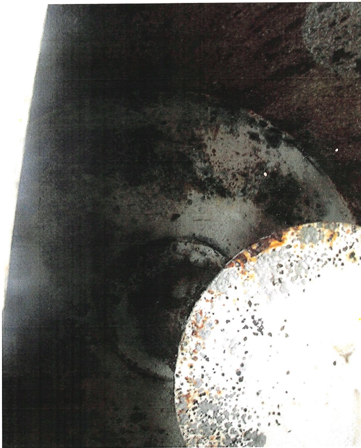
Photo shows the riser floor after all sediment has been removed. Pitting is present throughout the floor and milk stool cover.
