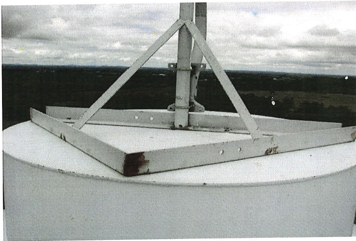
Photo shows an antennae mounted to the vent cover. The antennae should be moved to a stand-alone support welded to the roof cap plate to provide easier vent access.
