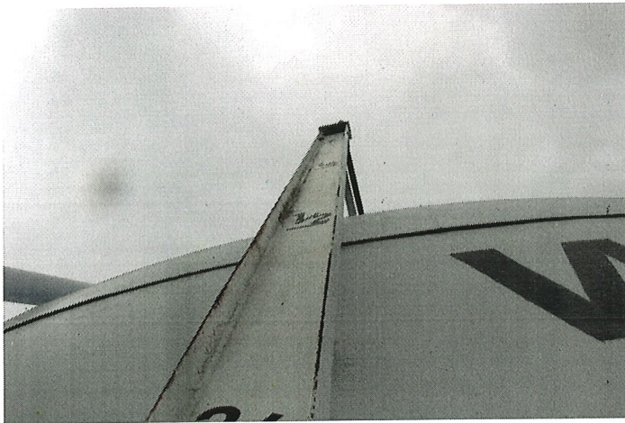
Photo shows the deficient water level indicator target board. The board should be removed if an active SCADA system is in place.
