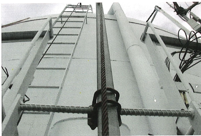
Photo shows the upper bracket for the tower ladder cable style climber safety device. The bracket should be lowered to allow a climber easier access to the balcony.
