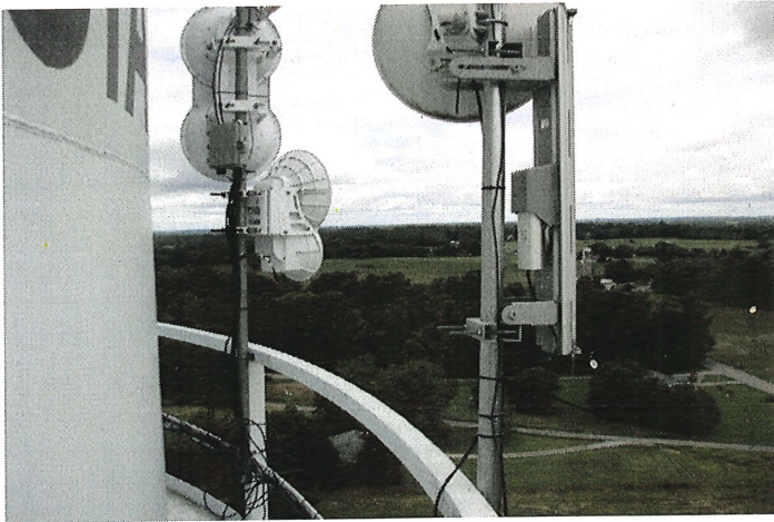
Photo shows two antennas mounted to the north section of the balcony handrail.
