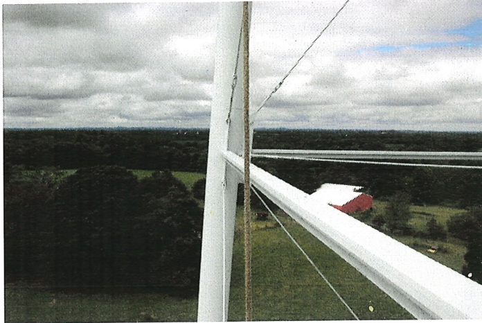
Photo shows the south facing upper strut. All member alignment is within tolerance.
