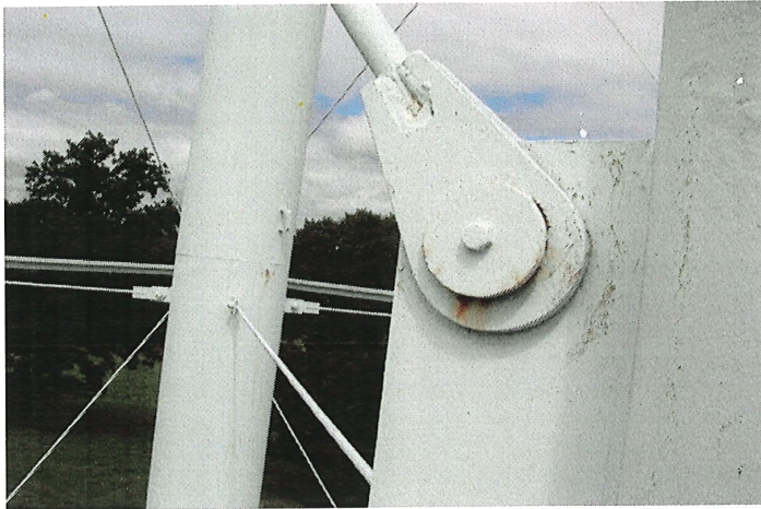
Photo shows crevice corrosion present along the southeast middle windage rod to leg pinned connection.
