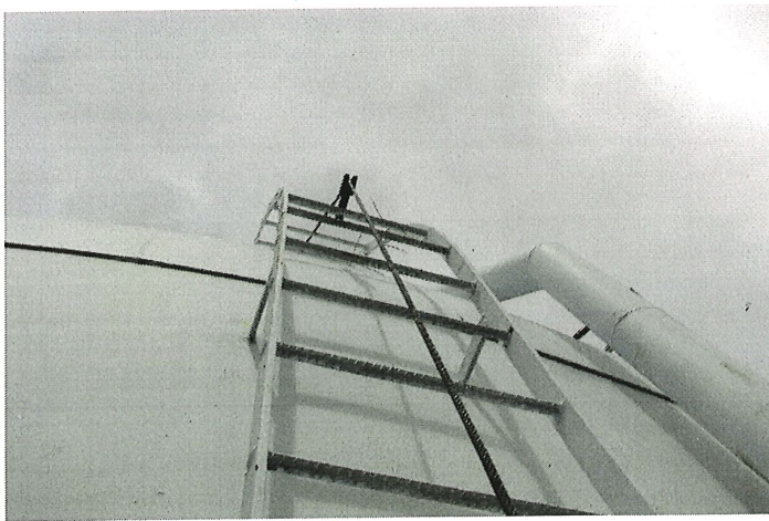
Photo shows the east section of the shell, roof ladder, and overflow pipe. The coating continues to protect the steel.
