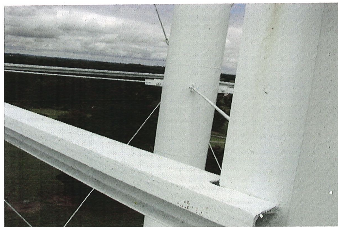
Photo shows minor rust bleed along the upper strut pinned connection point.
