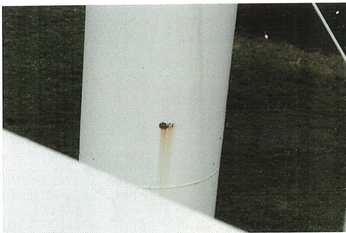
Photo shows an active corrosion cell present along the middle section of the riser.
