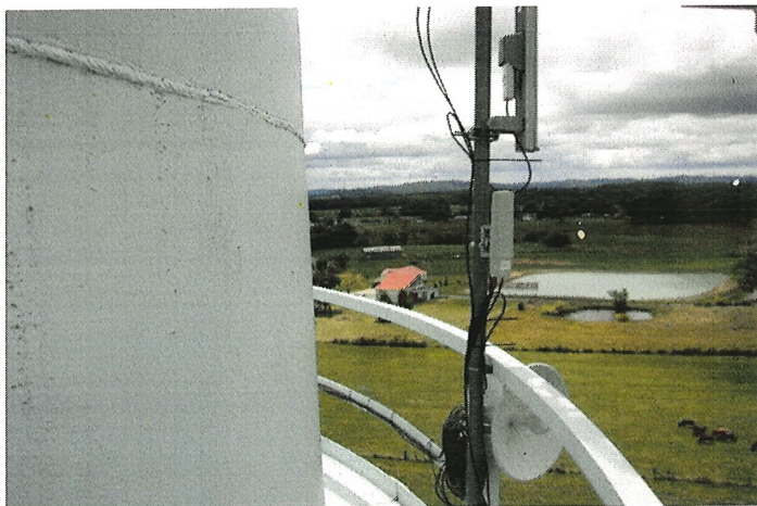
Photo shows an antennae mounted to the south section of the balcony handrail. Installing a roof corral and relocating all antennas should be considered.
