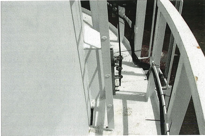
Photo shows the southeast section of the lower shell, balcony floor, and handrail. Small areas of localized corrosion can be seen.
