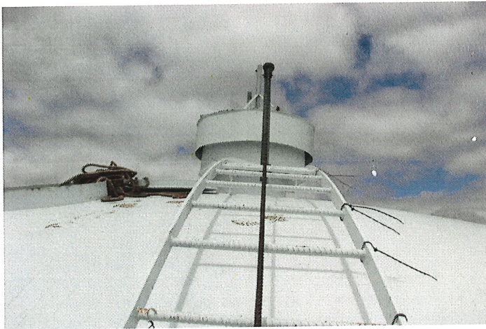
Photo shows the roof ladder equipped with a cable style climber safety device.
