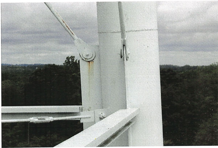
Photo shows crevice corrosion and rust bleed present along the northeast upper windage rod to leg pinned connection.
