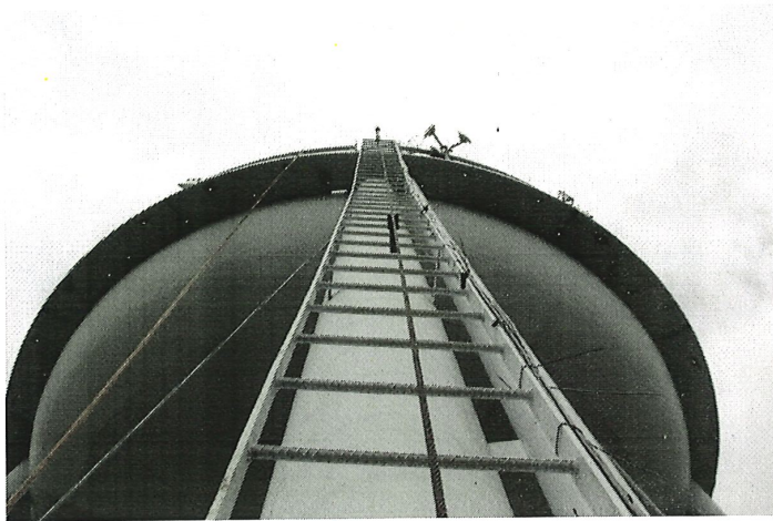
Photo shows the upper section of the tower ladder equipped with a cable style climber safety device.
