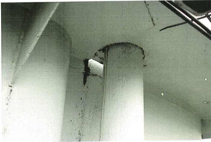
Photo shows the overflow pipe and underside of the balcony. Minor corrosion is present.
