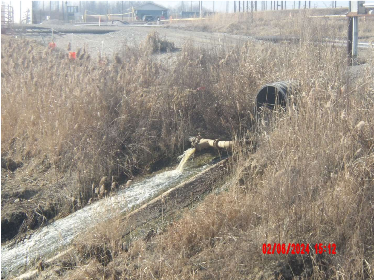
Water being discharged from filtered building
