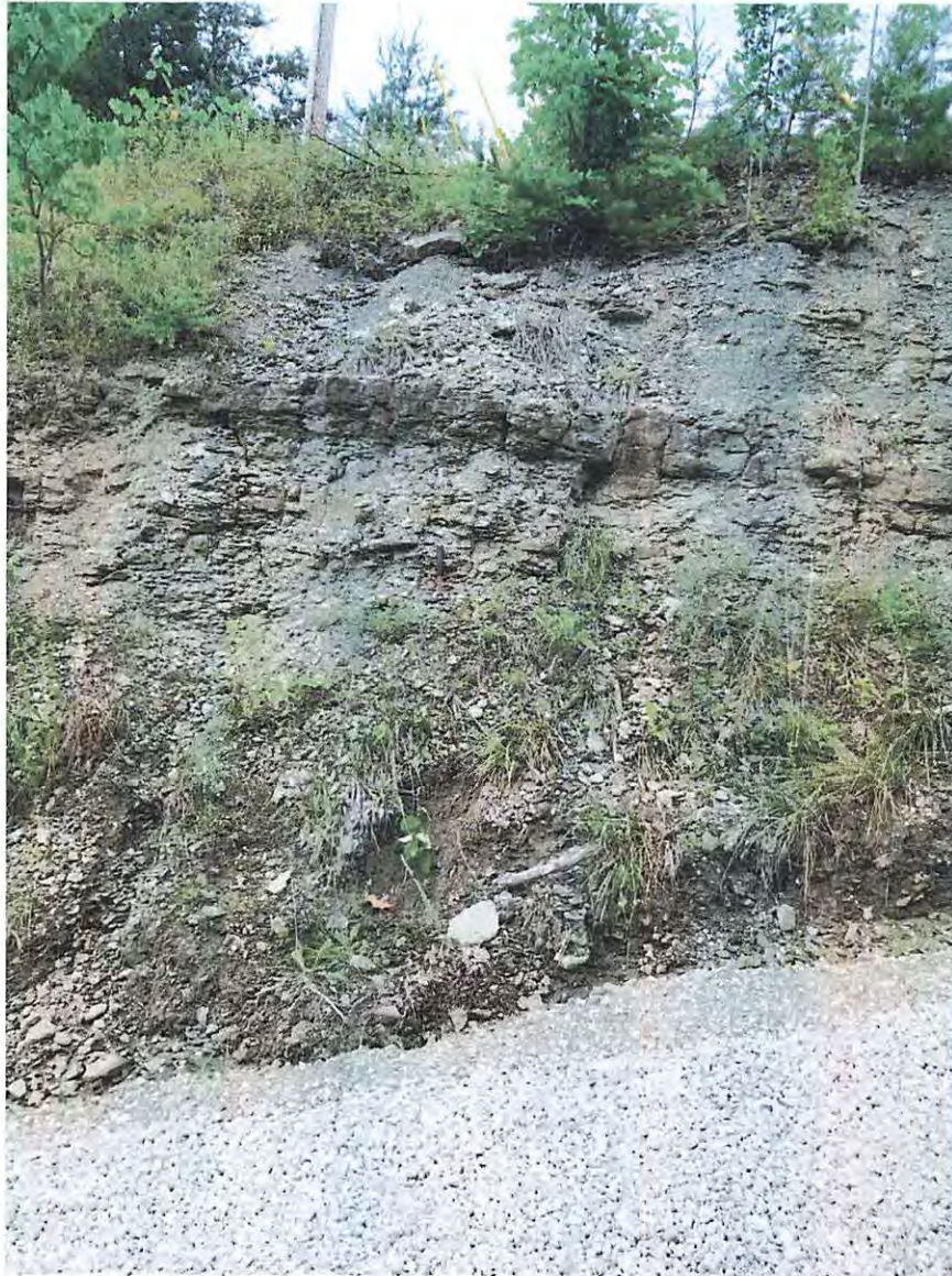
Photograph C – Access road highwall exposure showing rock to be encountered during foundation construction. Photo taken from access road facing west.
