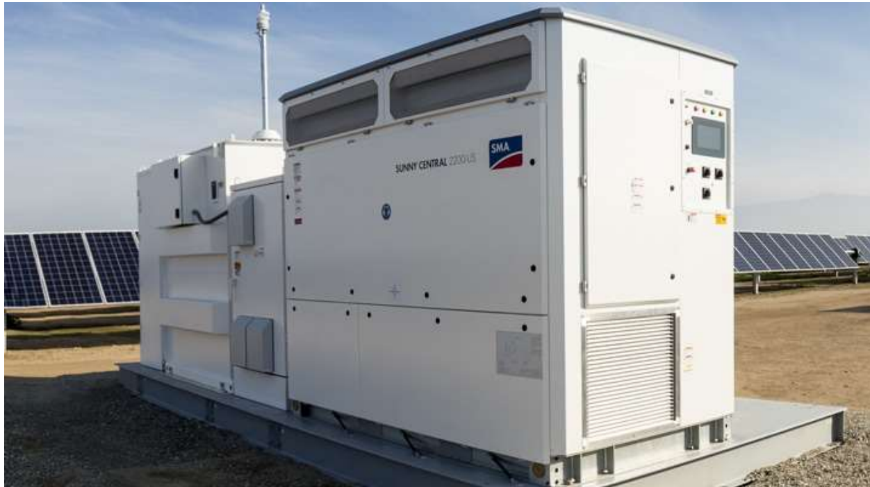
Picture (4) Industrial Solar Inverter 4
