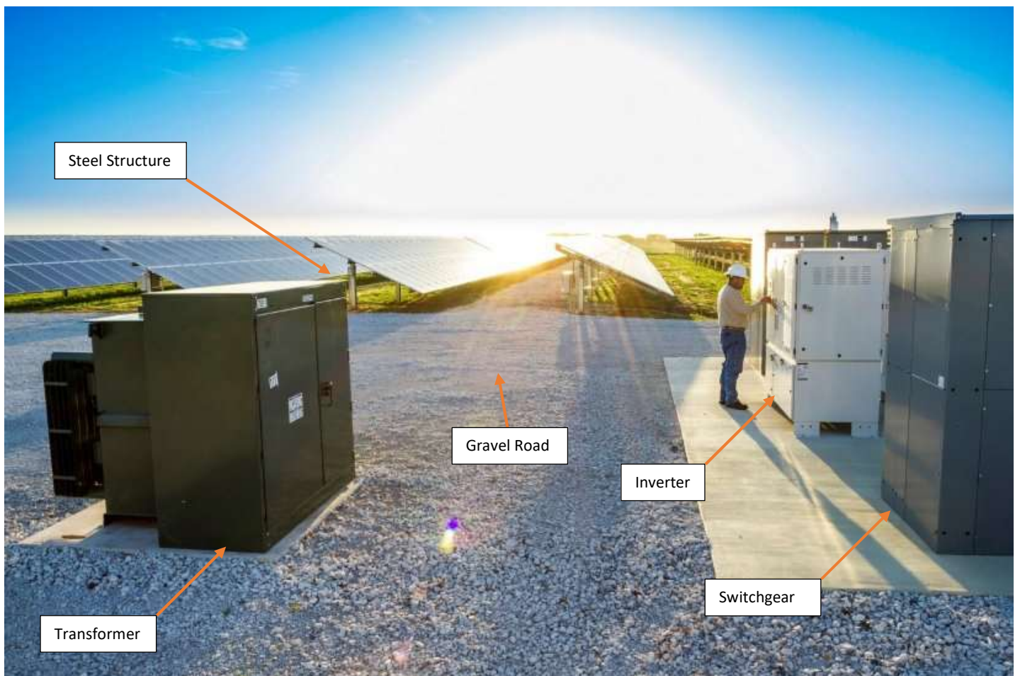
Picture (7) Steel & Concrete Structures of a 2MW Solar farm 7
