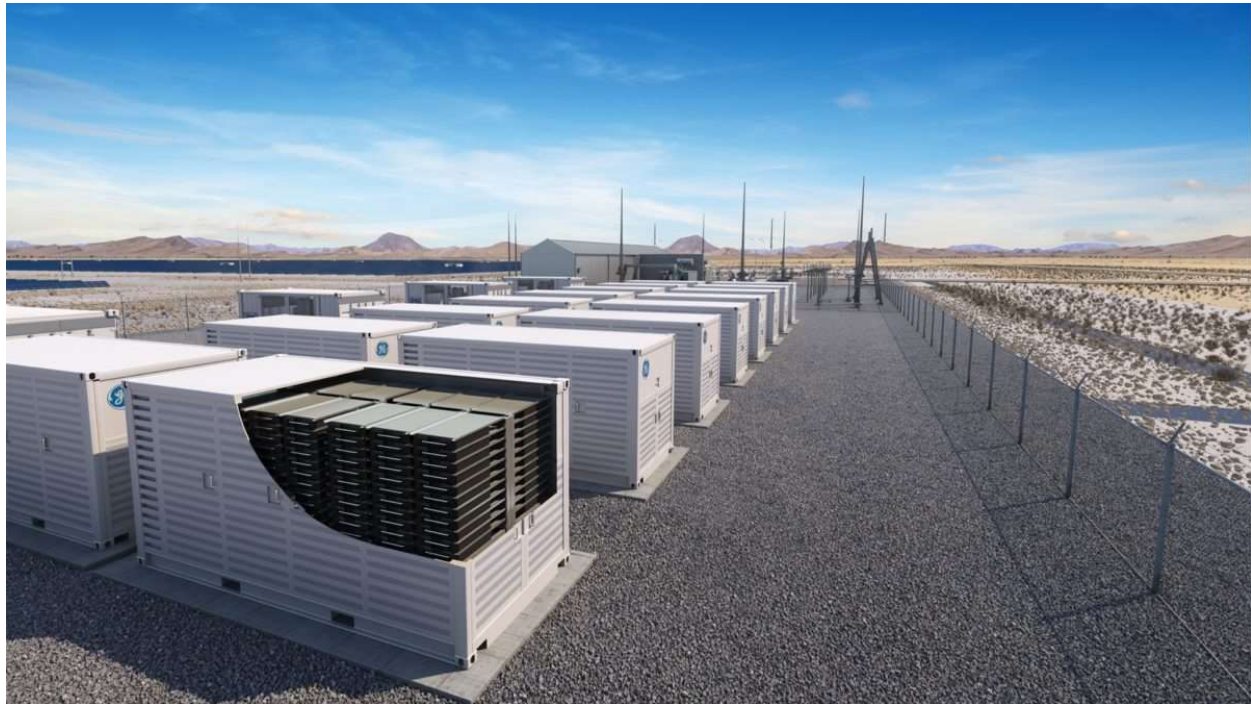
Picture (5) GE Industrial Battery 5
