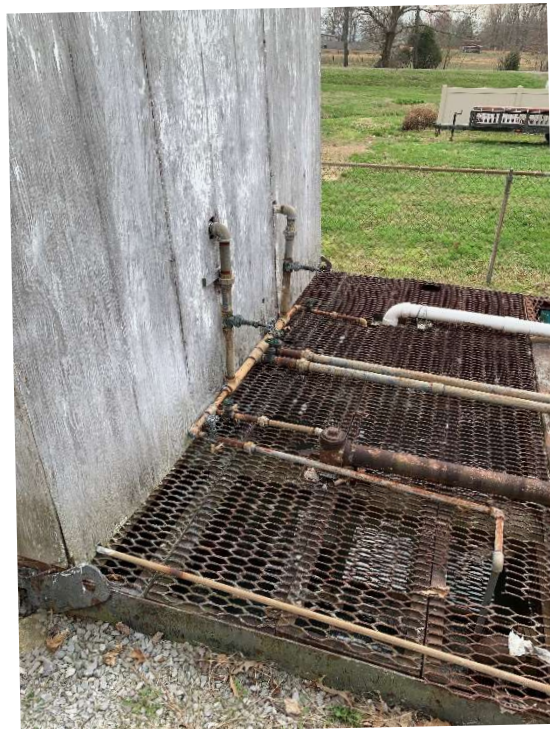
Secondary Clarifier and Air Header from Blower Shed
