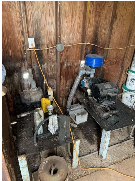
View Inside Blower Shed
