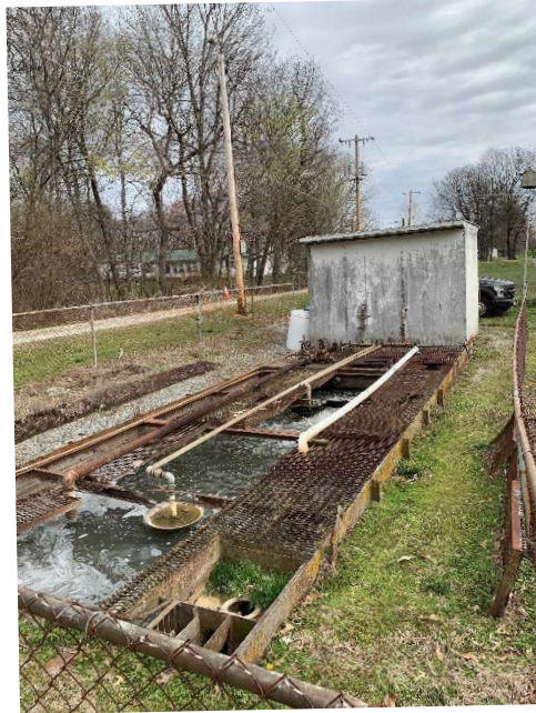
View of Existing Wastewater Treatment Facility
