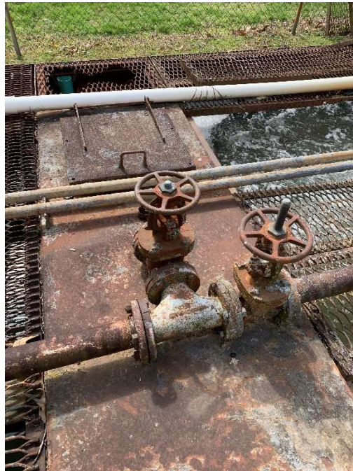
Secondary Clarifier with Return Lines
