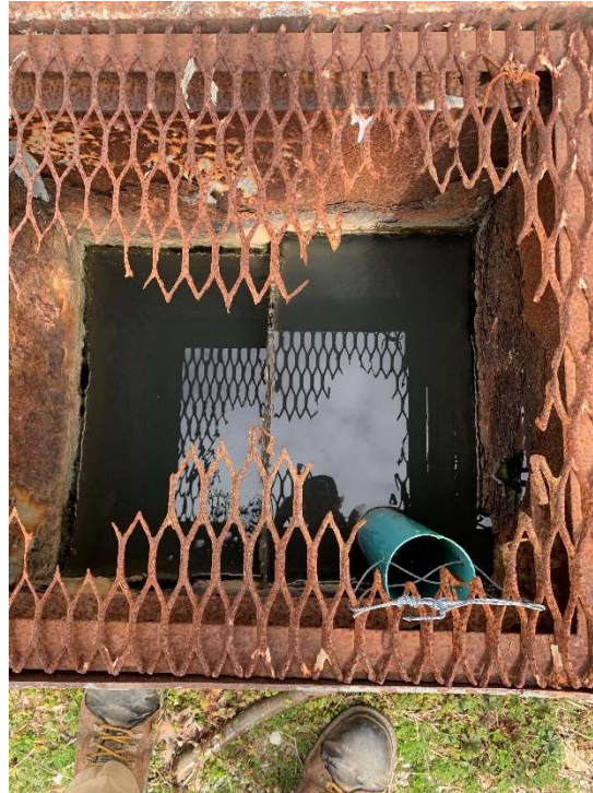
Disinfection Basin with Baffle Wall
