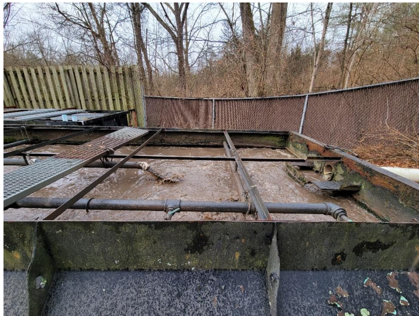
RAS and Influent Lines
