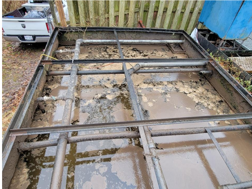
RAS, Scum, and Air Header Lines
