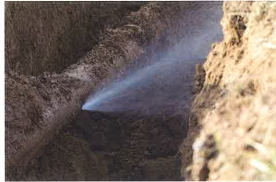
Figure 9: Typical leak we expect to find in this project.
